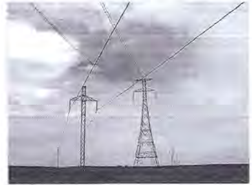
Two HVDC lines cross. Square Butte is the line of towers on the left. The CU tower line is on the right, with each of its two conductors formed of two sub-conductors in a horizontal configuration.
