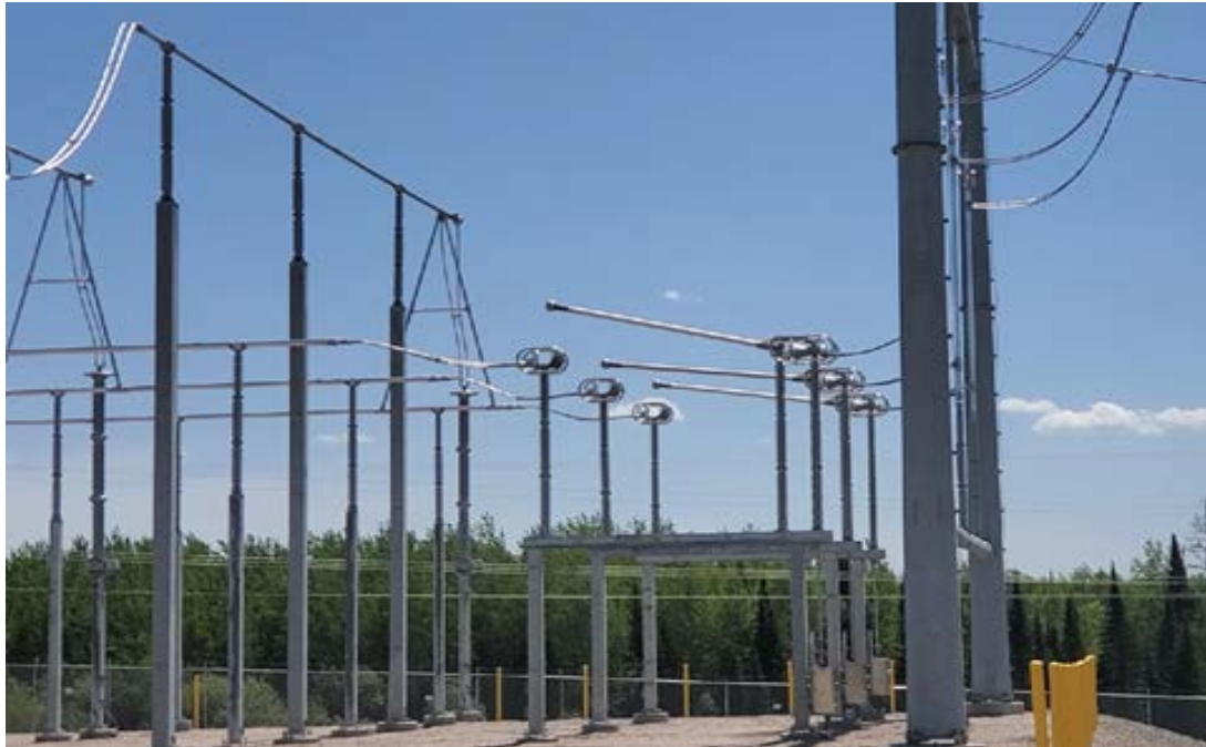
Substation switch closing
