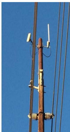
Figure 46: WiMAX Portion of the FAN on a Distribution Pole
