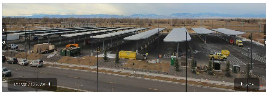
Figure 64: 1.3 MW Carport Solar Installation
