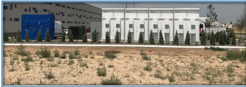
Figure 65: 1 MW Battery System
