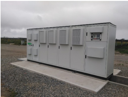
Photo 2 Typical Inverter Skid
