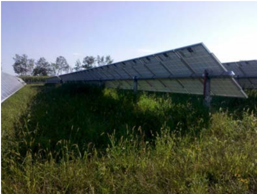
Photo 1 Typical Solar Array and Tracking System
