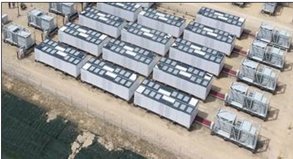
Figure 4: Representative ESS Units
