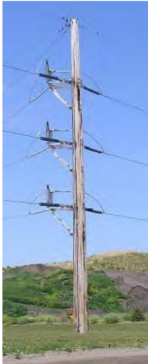
Typical Switch Structure
