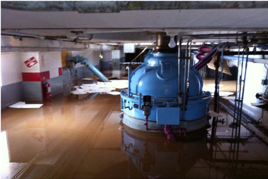
Figure 4. Thomson Basement After the June 2012 Flood
