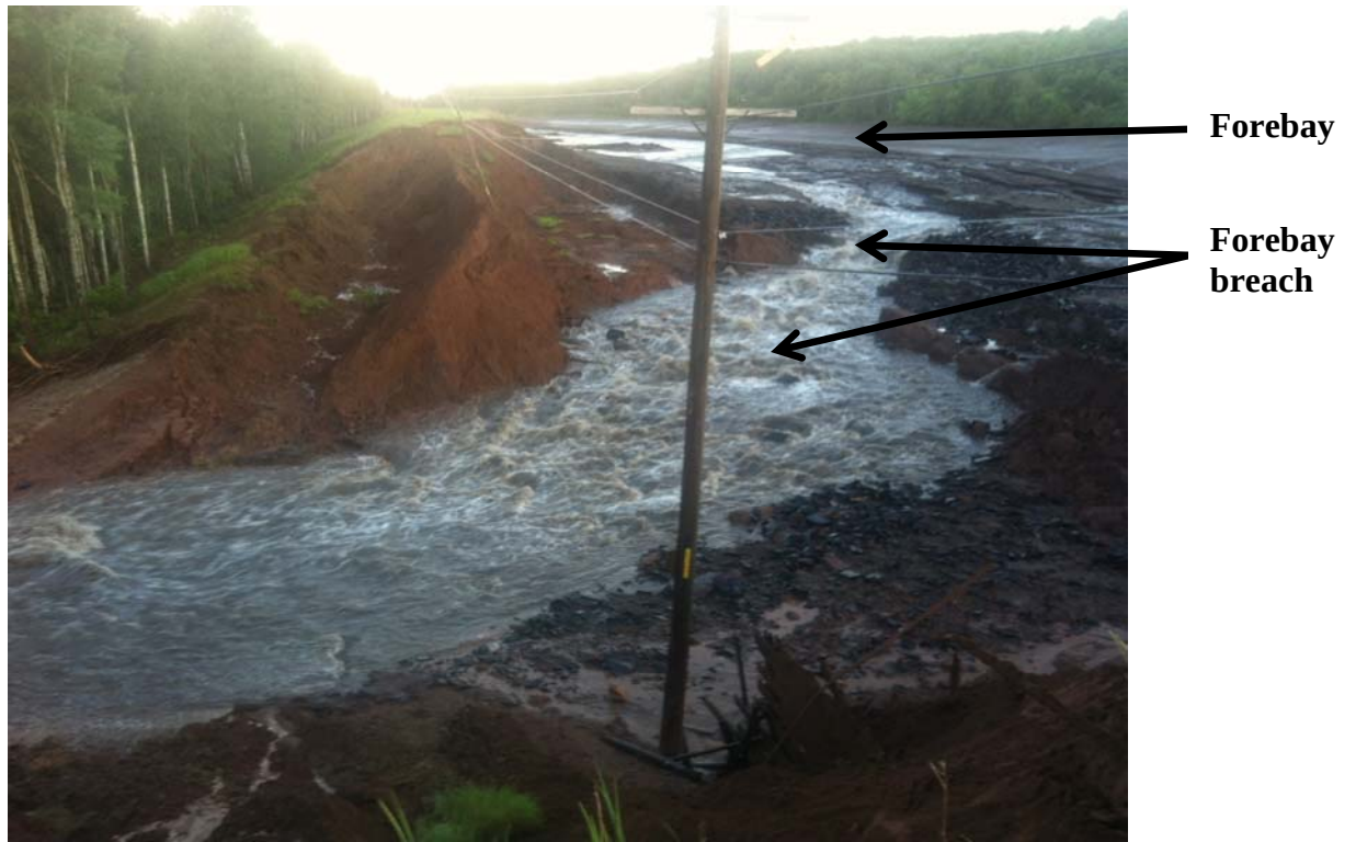
Figure 2. Forebay Breach After the June 2012 Flood
