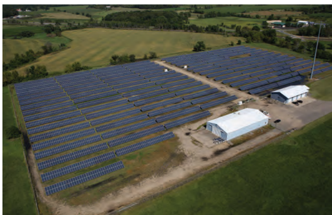
The 2.25 MW Dickinson Solar Project serves Wright-Hennepin Cooperative Electric Association's membership.
