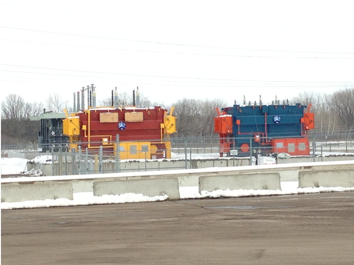
New 1R and 2R Transformers Onsite
