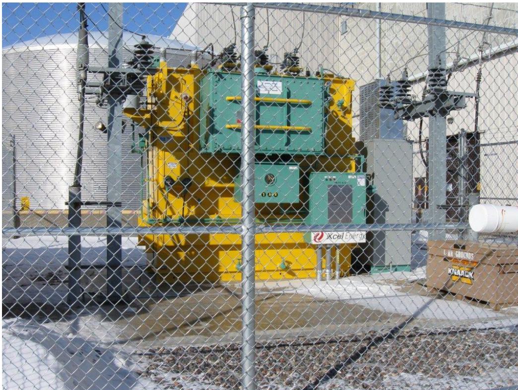
New 1AR Transformer
