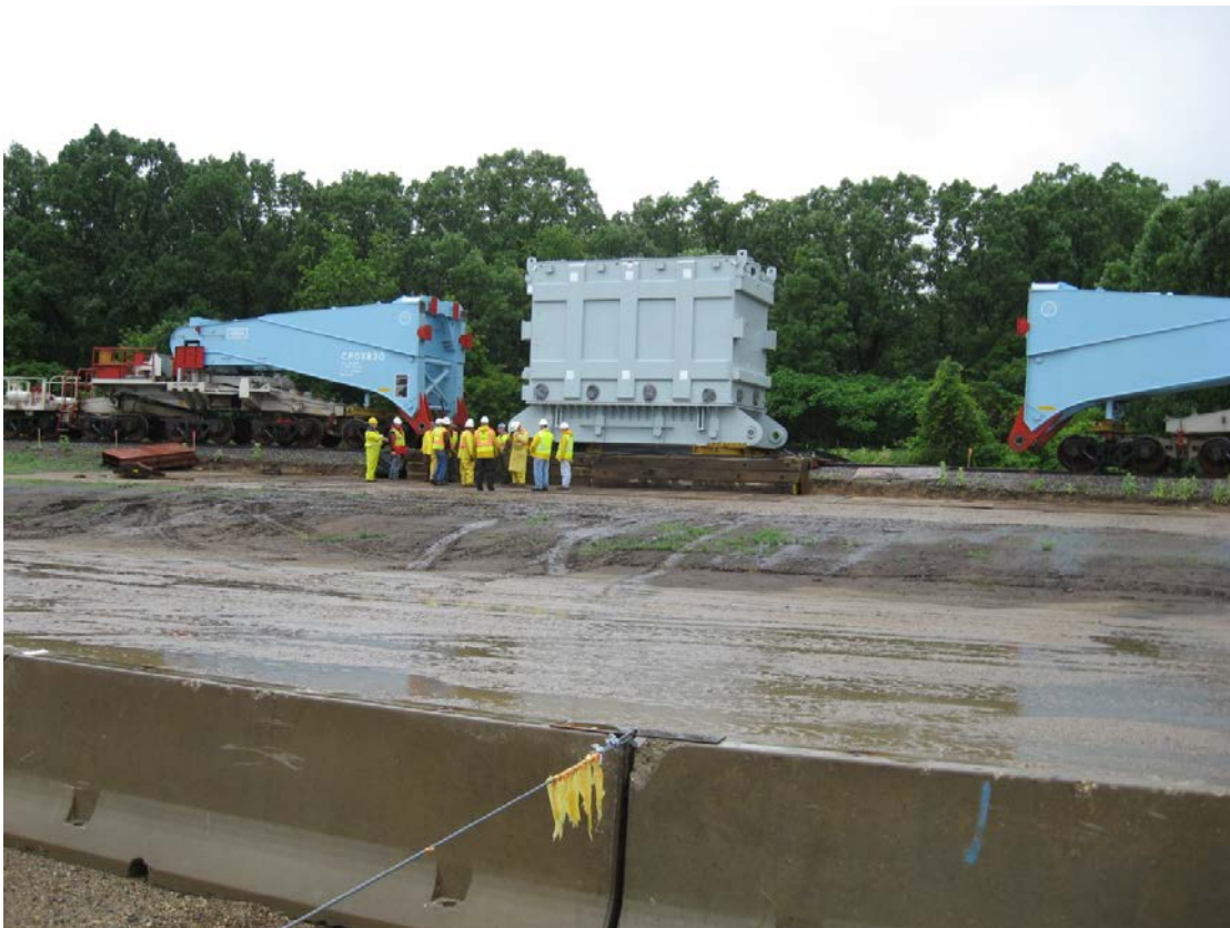
Main Power Transformer Arrival Onsite
