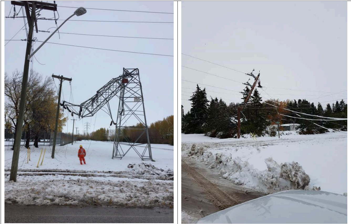
Figure 5: Damage from October Storm in Manitoba
