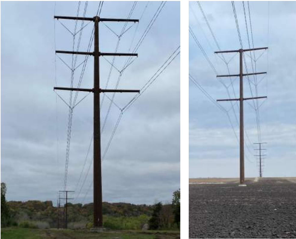
Figure 3-3 Example Double-Circuit, Monopole 345 kV Structures with V-String Insulators
