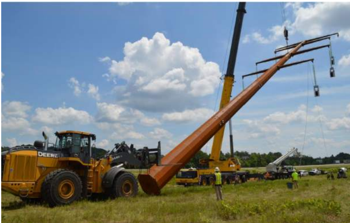
Structures are assembled before being lifted into place with a crane. Source: reference (7)
