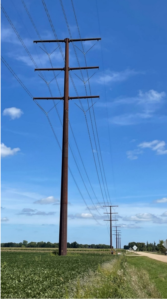
Double-circuit tangent structure
