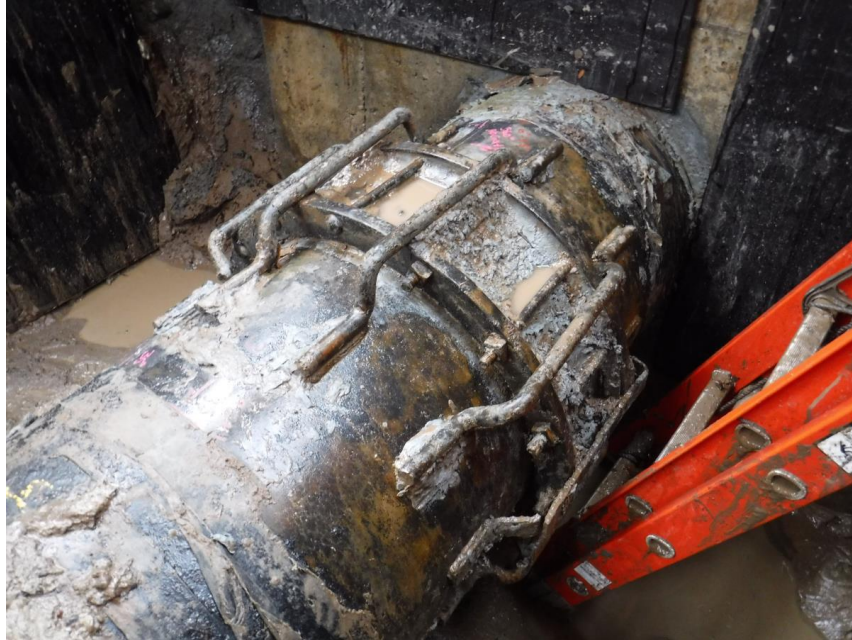
Coupling with broken support bars; 8 out of 9 failed.
