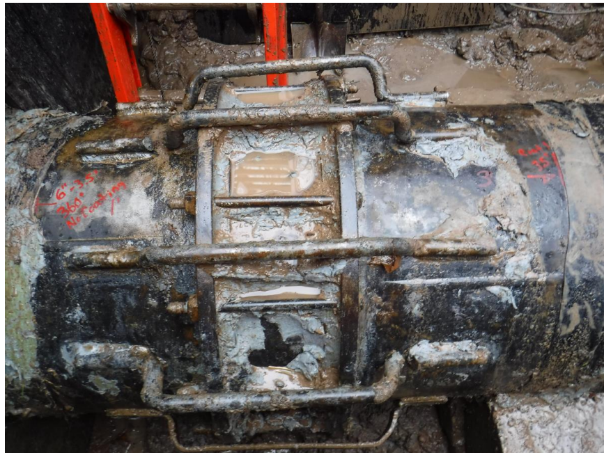
Coating failure from 6" to 3.5"
