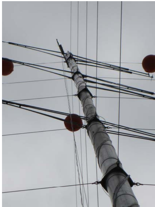
Photo2. Tower 2 50m microphone on tower (tower 3 utilizes same system).
