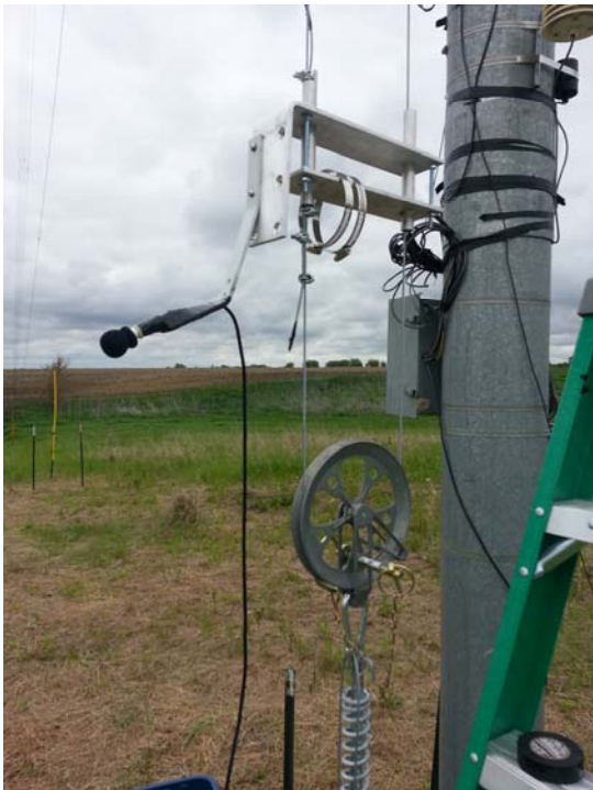
Photo 1. Tower 2 pulley assembly (tower 3 utilizes same system).
