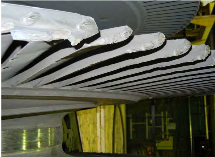
Fig. 68. Photograph of turbine end L-3 stage blading on low pressure turbine "B" rotor showing damage to covers and missing covers.
