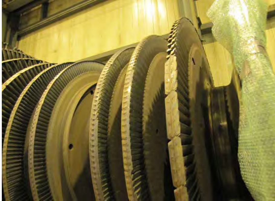
Fig. 66. Photograph of turbine end of low pressure turbine "B" rotor showing damage to L-2, L-3 and L-4 stage blade covers.
