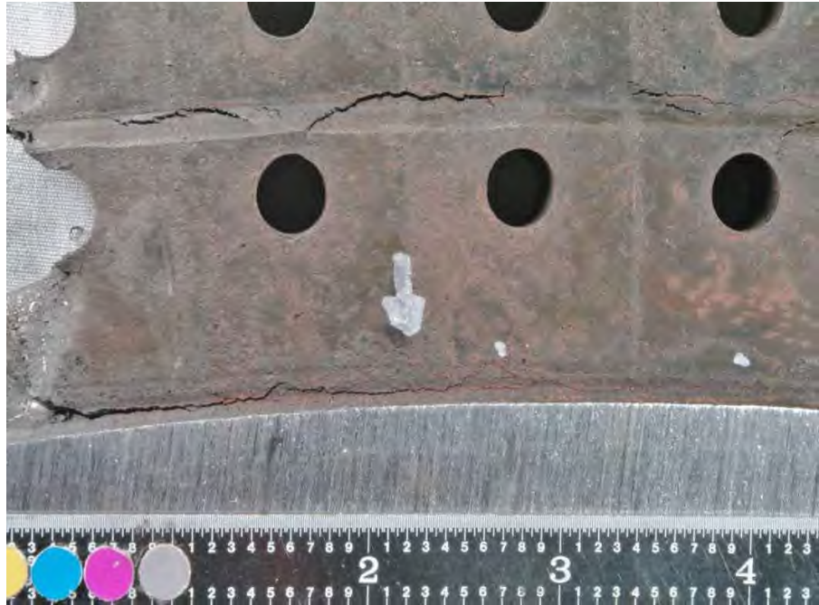
Fig 158. Close-up of SID 14875 subsegment "C4" crack 1 identified in Fig. 155, viewed from inlet side.
