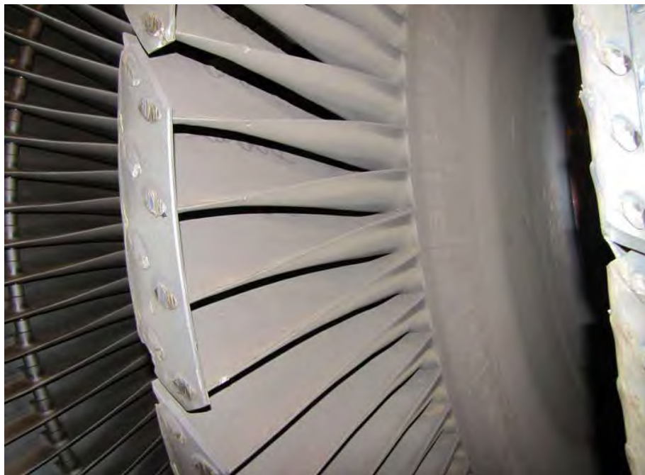
Fig. 49. Generator end of low pressure turbine "A" showing extent of rub damage on L-2 blade covers and tenons.
