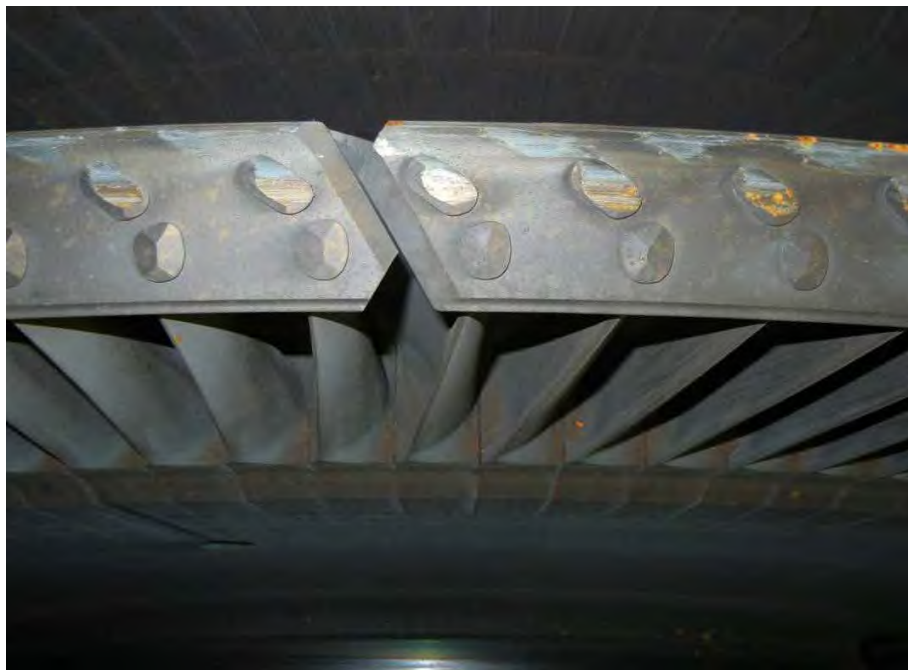
Fig. 51. Close-up of low pressure turbine "A" turbine end L-3 stage blade covers showing extent of rub damage.
