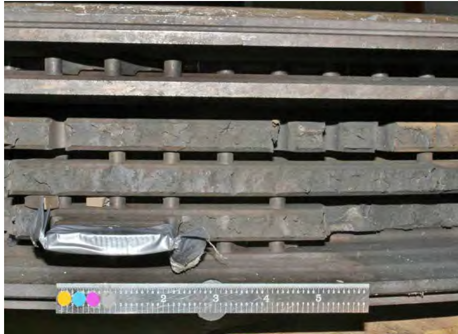
Fig. 124. Close-up photograph of fractures through internal finger pinned blade attachments in low pressure turbine "B" L-1 disk rim.
