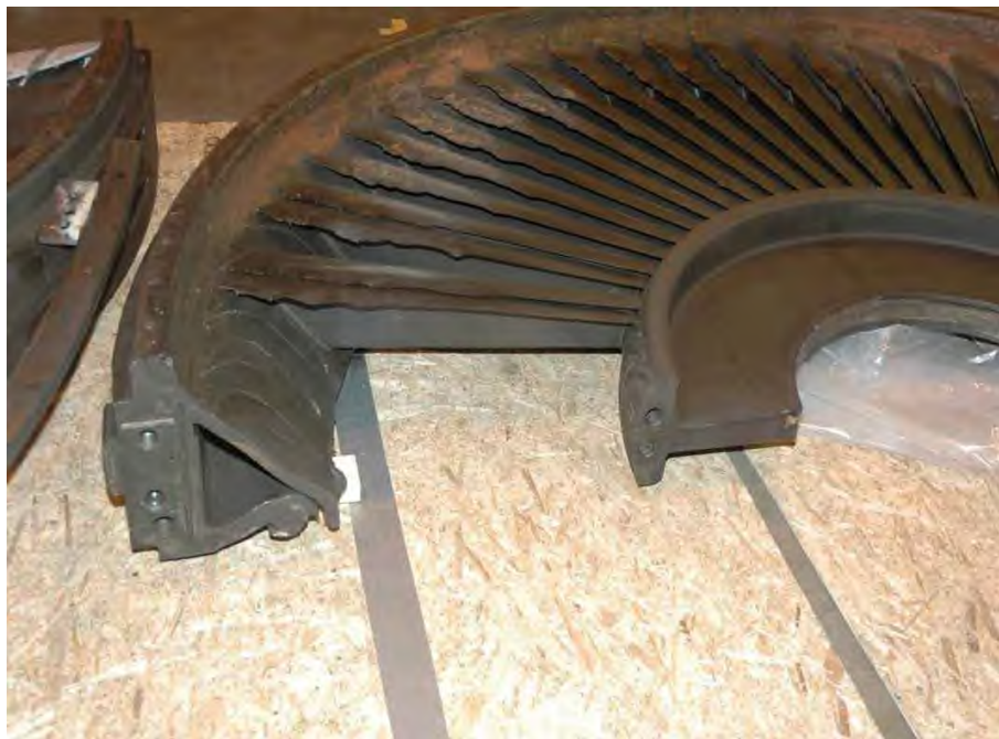
Fig. 77. Photograph of turbine end last stage diaphragm from low pressure turbine "B" rotor showing extent of damage.
