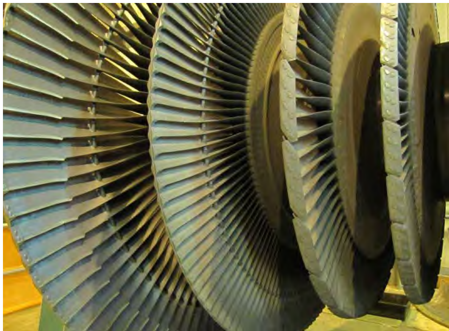
Fig. 47. Photograph of generator end of low pressure turbine "A" rotor shown in Fig. 44..
