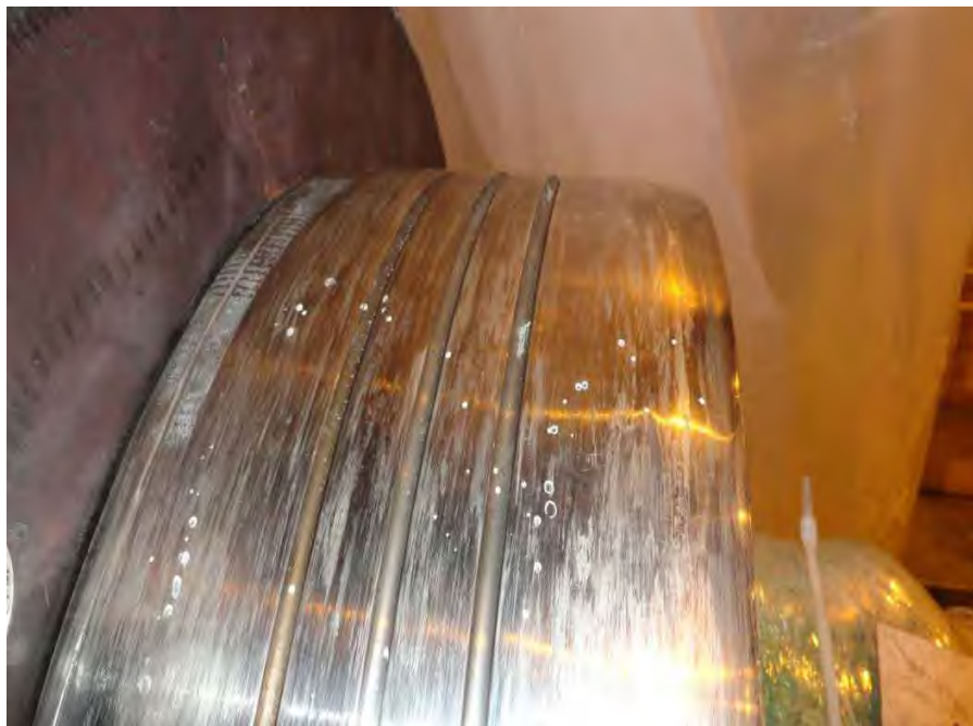
Fig. 114. Generator rotor CE oil seal journal showing extent of rub damage.
