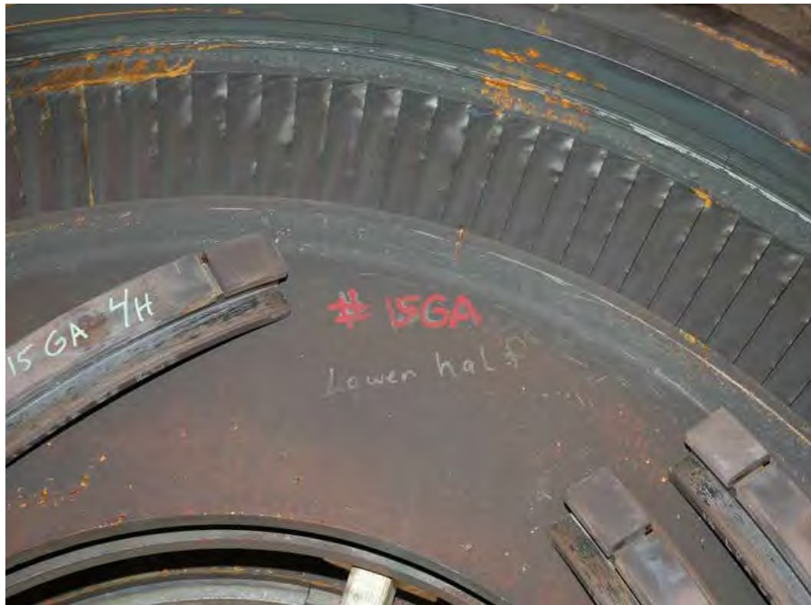
Fig. 53 Close-up of generator end L-4 diaphragm from low pressure turbine "A" showing rub damage to vanes.
