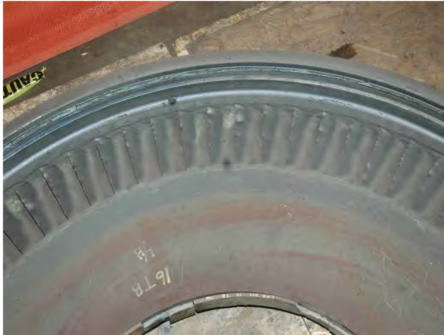
Fig. 80. Photograph of low pressure turbine "B" turbine end L-3 stage diaphragm showing extent of impact damage.
