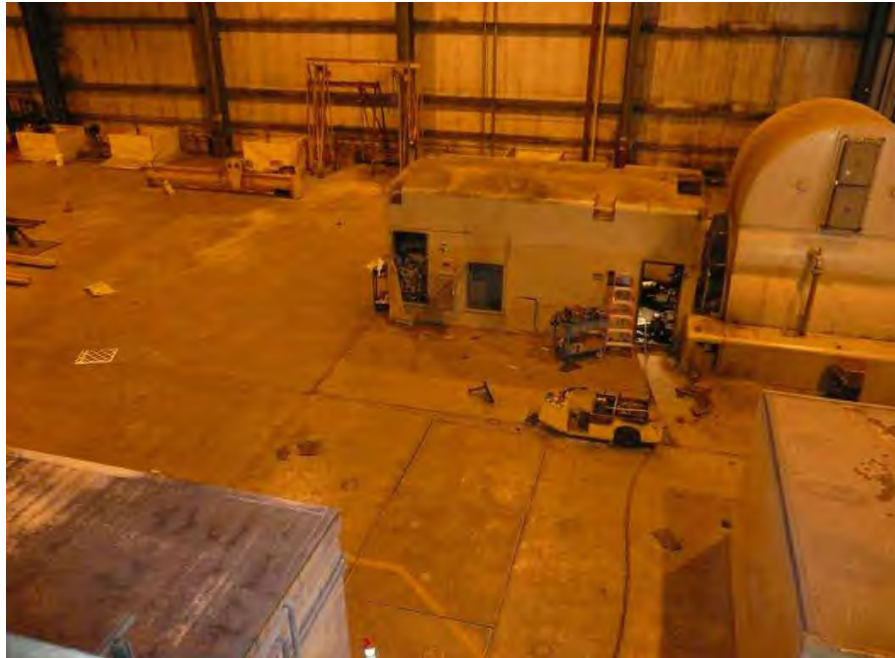
Fig. 4. Photograph of Sherco Unit 3 steam turbine generator after the event of November 19, 2011.
