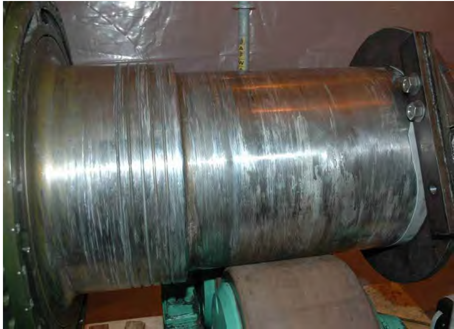
Fig. 112. Generator rotor rub damage.
