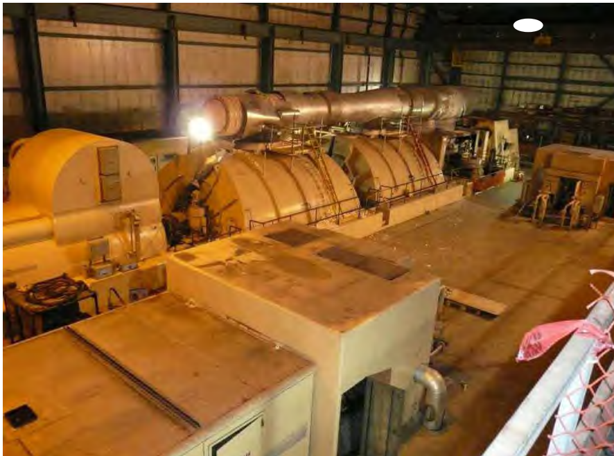
Fig. 2. Photograph of Sherco Unit 3 steam turbine generator after the event of November 19, 2011
