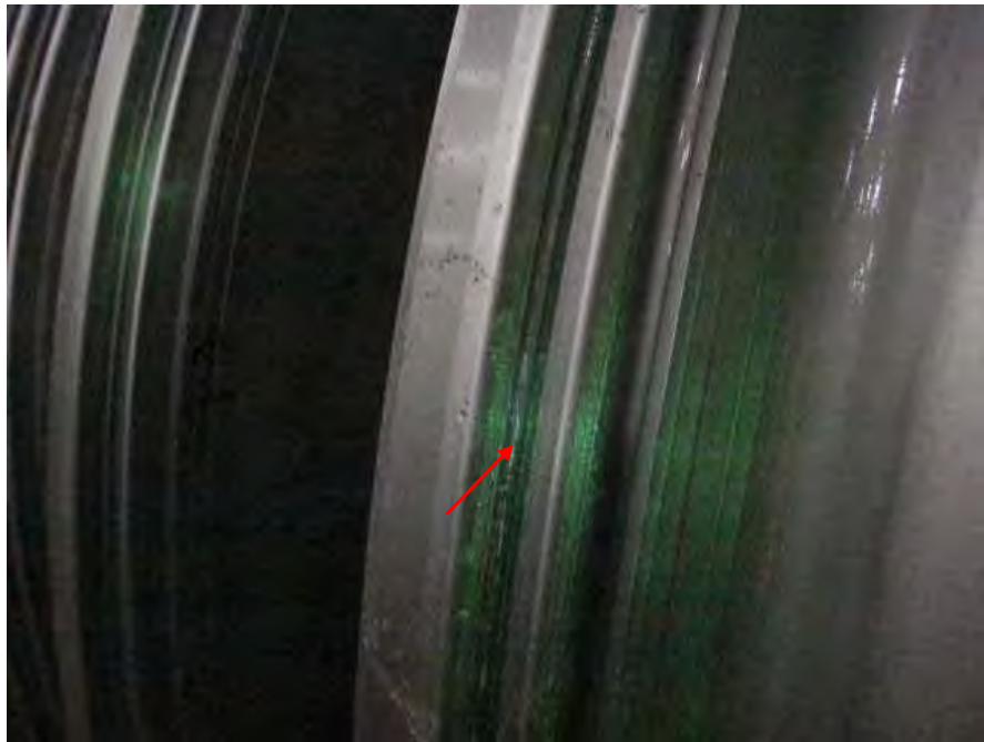
Fig. 97. Close-up blacklight photograph of low pressure turbine "A" generator end L-4 stage disk on inlet side of the blade dovetail showing indication (arrow).
