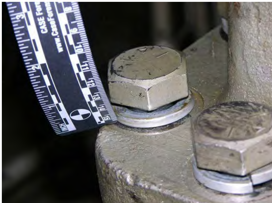
Fig. 10. Photograph of an outer casing fastener from the Sherco Unit 3 steam turbine generator after the event of November 19, 2011.
