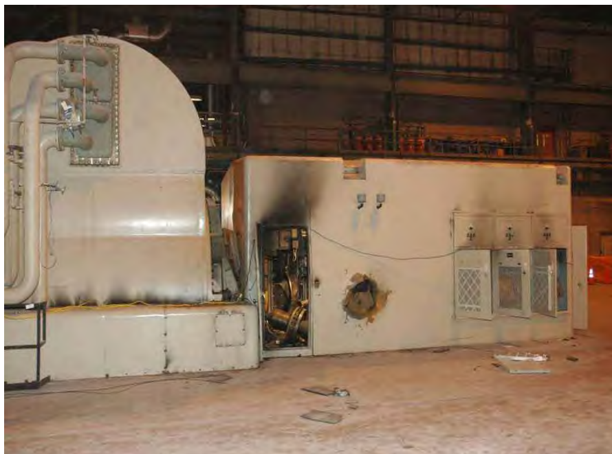
Fig. 7. Photograph of Sherco Unit 3 steam turbine generator at exciter end after event of November 19, 2011.
