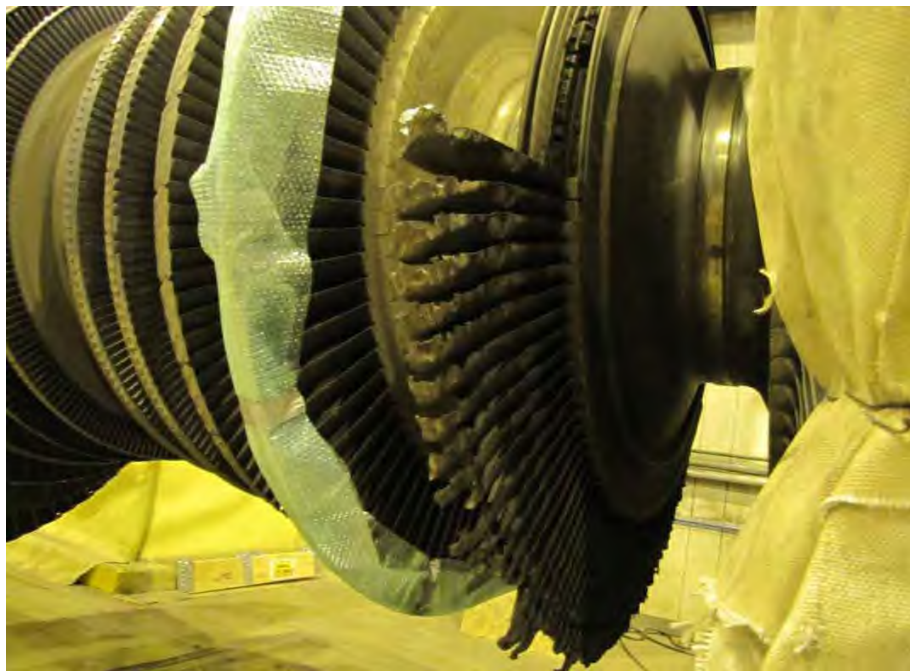
Fig. 57. Close-up of fractured turbine end L-1 stage disk of the low pressure turbine "B" rotor shown in Fig. 55.
