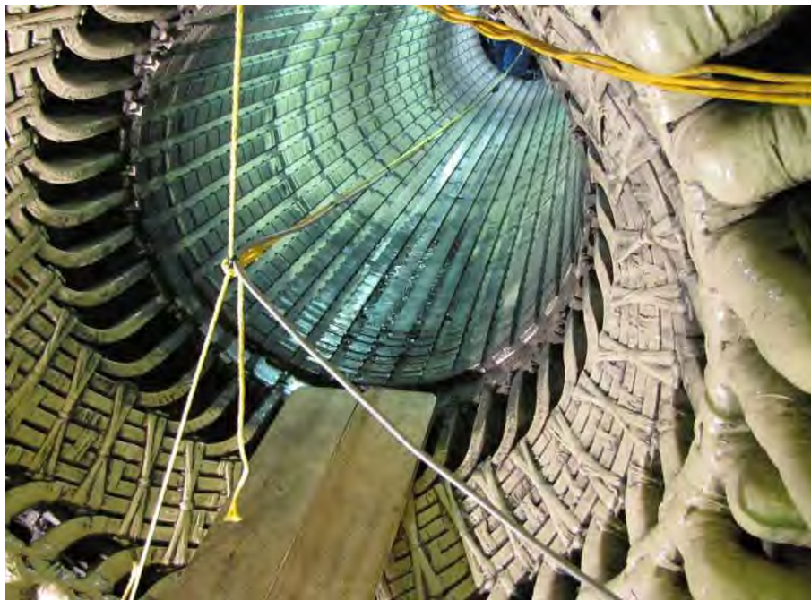
Fig. 111. Photograph of generator stator showing extent of rub damage.
