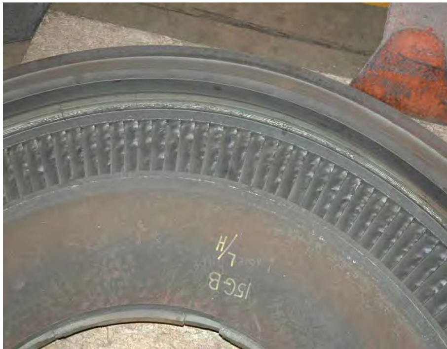
Fig. 81. Photograph of low pressure turbine "B" generator end L-4 stage diaphragm showing extent of impact damage to vane airfoils.
