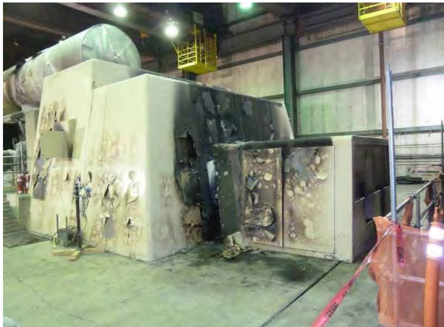
Fig. 5 Photograph of high pressure end of Sherco Unit 3 steam turbine generator after the event of November 19, 2011.
