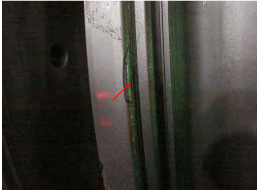
Fig. 96. Close-up blacklight photograph of low pressure turbine "A" generator end L-4 stage disk on exit side of the blade dovetail showing indication (arrow).
