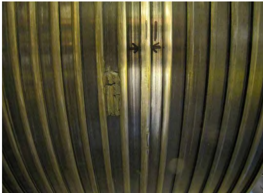
Fig. 35. Close-up photograph of Intermediate Pressure Turbine showing rub damage on seal surface.
