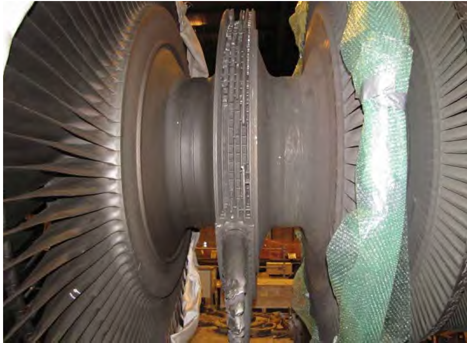
Fig. 58. Close-up of fractured disk section of turbine end L-1 stage on low Pressure turbine "B" rotor shown in Fig. 55.
