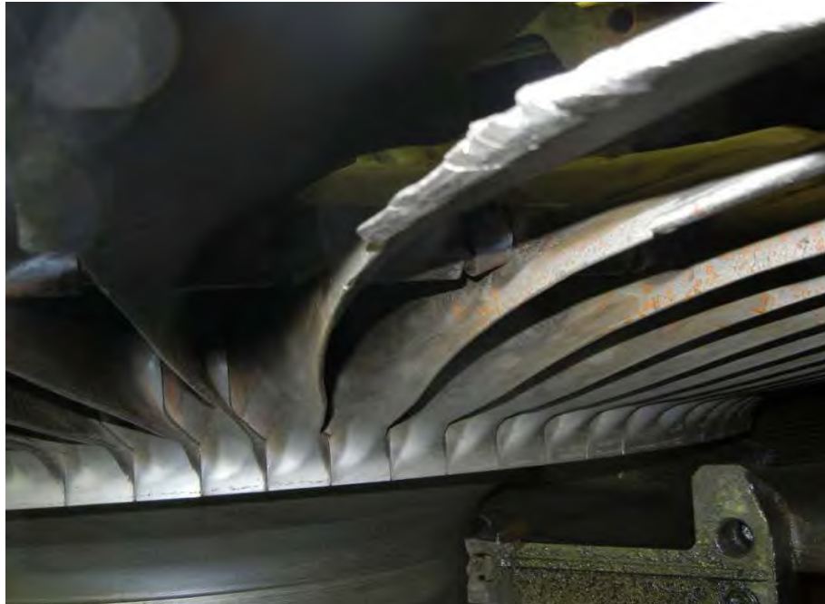
Fig. 74. Photograph of low pressure turbine "B" generator end last stage blades showing damage to stellite leading edges.
