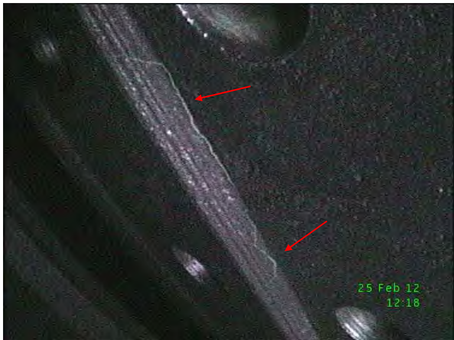
Fig. 91 Close-up blacklight photograph of low pressure turbine "A" L-1 disk rim showing MPI indication (arrows) in finger-root attachment.
