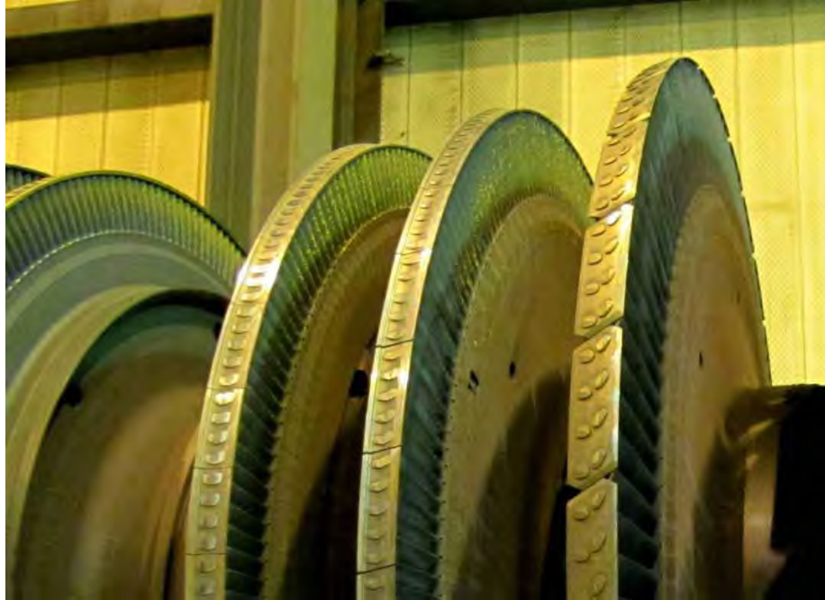
Fig 52. Close-up of low pressure turbine "A" showing rub damage to trailing edges of turbine end L-5 and L-4 blades and leading edges of generator end L-5 stage blades.
