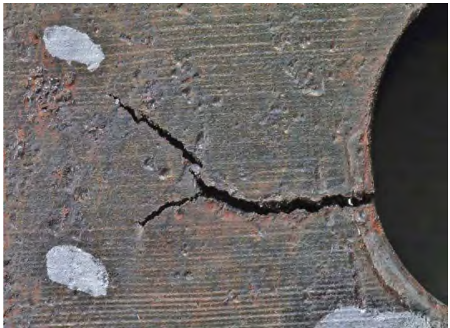
Fig 165. Close-up of SID 14875 subsegment "C4" crack No. 3 shown in Fig. 164, viewed from inlet side.
