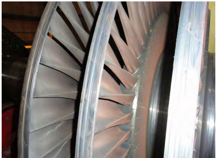
Fig. 33 Close-up of intermediate pressure turbine rotor shown in Fig. 31 showing moderate to heavy rub damage on blade integral shrouds.
