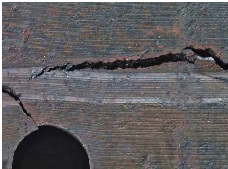
Fig 162. Close-up of SID 14875 subsegment "C4" crack No. 2 shown in Fig. 161, viewed from inlet side.
