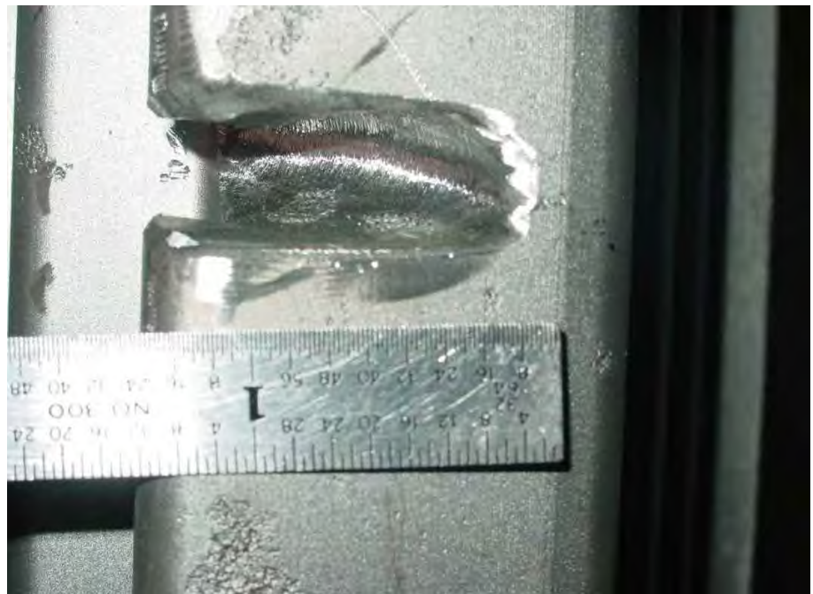
Fig. 101. Close-up photograph of low pressure turbine "A" generator end L-2 stage disk rim showing excavation of indication at 330° location. Viewed from top.
