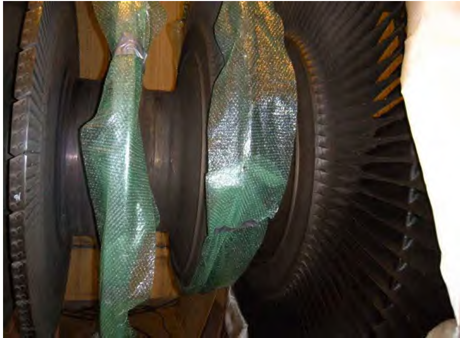
Fig. 82. Photograph of low pressure turbine "B" L-1 stage fractured disk rim with bubble wrap protection.
