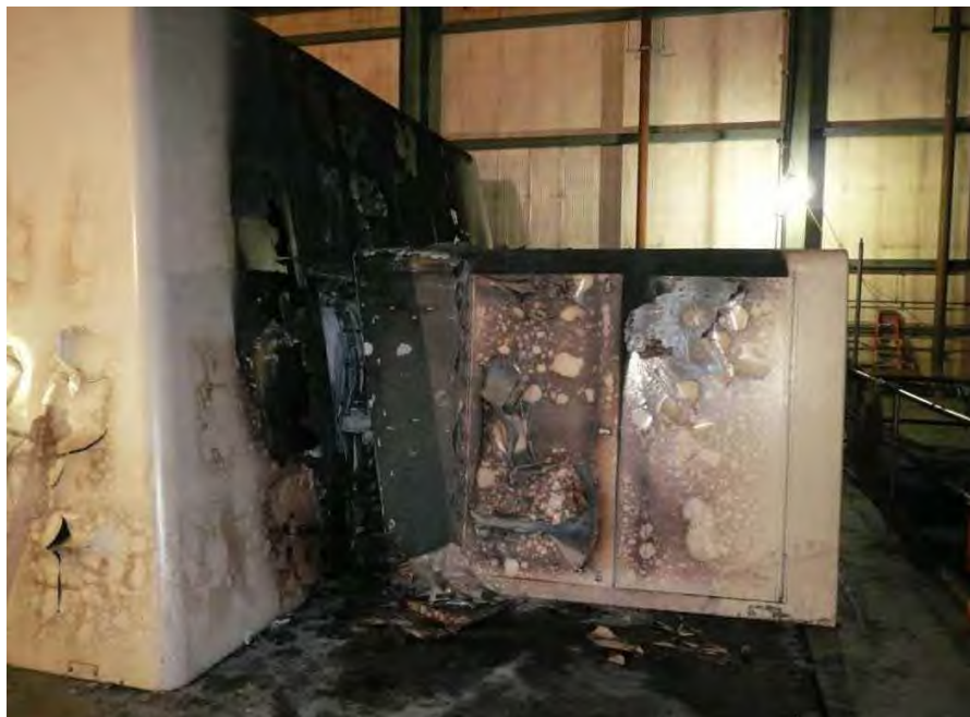
Fig. 6. Photograph of high pressure end of Sherco Unit 3 steam turbine generator after event of November 19, 2011.
