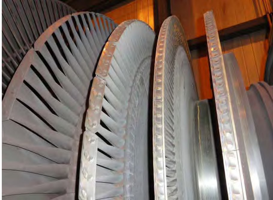
Fig. 48. Generator end of low pressure turbine "A" showing extent of rub damage on L-3, L-4 and L-5 blade covers and tenons.
