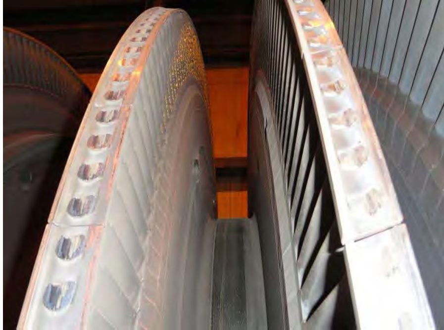
Fig. 50. Low pressure turbine "A" turbine end showing extent of rub damage on L-4 and L-5 blade covers and tenons.
