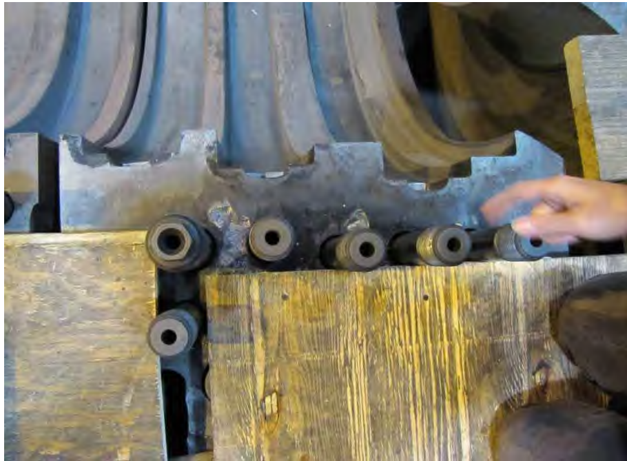
Fig. 27. Close-up of melted areas on intermediate pressure turbine inner casing, shown in Fig. 26, after removal of rotor and diaphragms.
