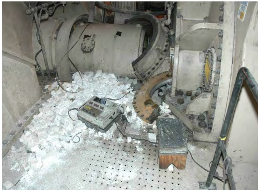
Fig. 9. Photograph of damaged coupling cover between the low pressure turbines of Sherco Unit 3 steam turbine generator after event of November 19, 2011.
