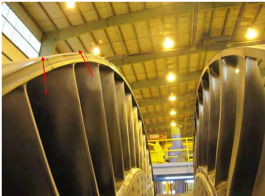
Fig. 15. Close-up of high pressure rotor shown in Fig. 12 showing rub damage (arrows) on blade integral shrouds.
