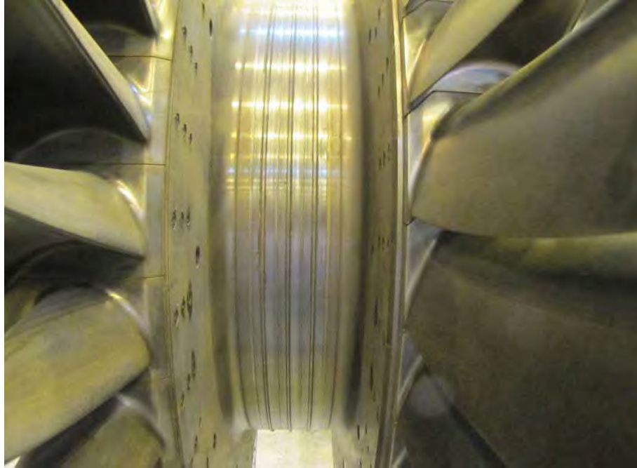
Fig. 16. Photograph of high pressure rotor shown in Fig. 12 showing light rub damage to interstage seal areas.
