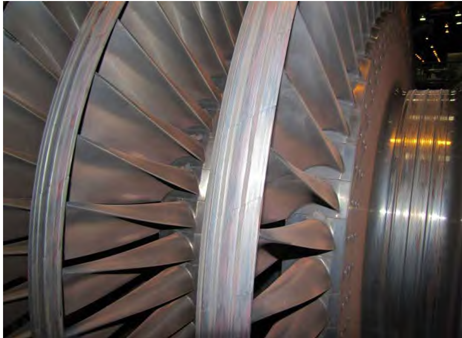
Fig. 32. Close-up of intermediate pressure turbine rotor shown in Fig. 31 showing moderate to heavy rub damage on blade integral shrouds.
