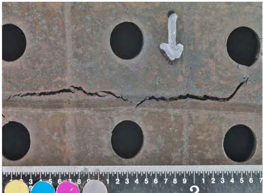
Fig 161. Close-up of SID 14875 subsegment "C4" crack No. 2 identified in Fig. 155, viewed from inlet side.
