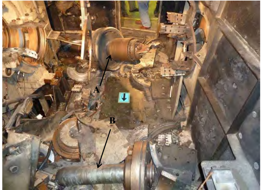
Fig. 104. Photograph of exciter doghouse showing portion of fractured generator shaft (arrow A) and portion of fractured exciter shaft (arrow B).
