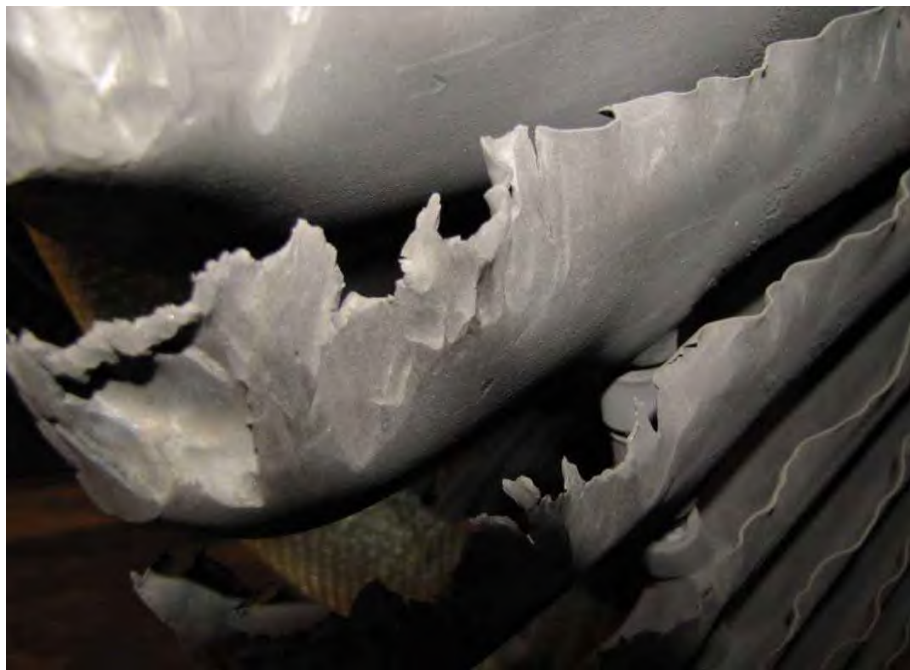
Fig. 61. Close-up photograph of turbine end L-1 stage blades from low pressure turbine "B" rotor shown in Fig. 55.
