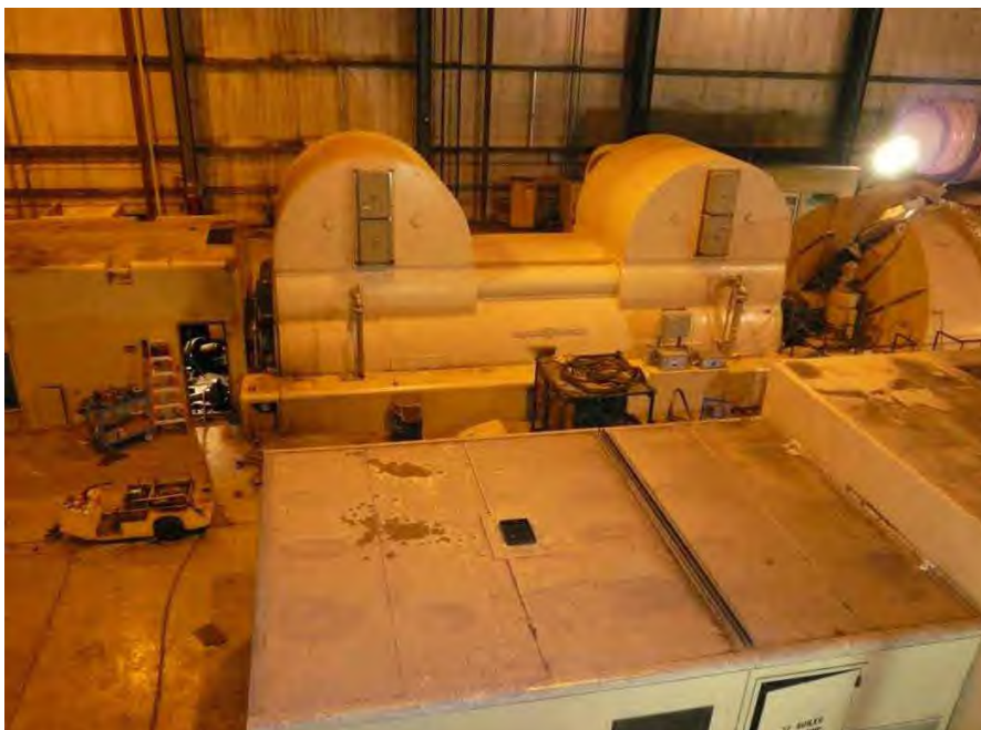
Fig. 3. Photograph of Sherco Unit 3 steam turbine generator after the event of November 19, 2011.
