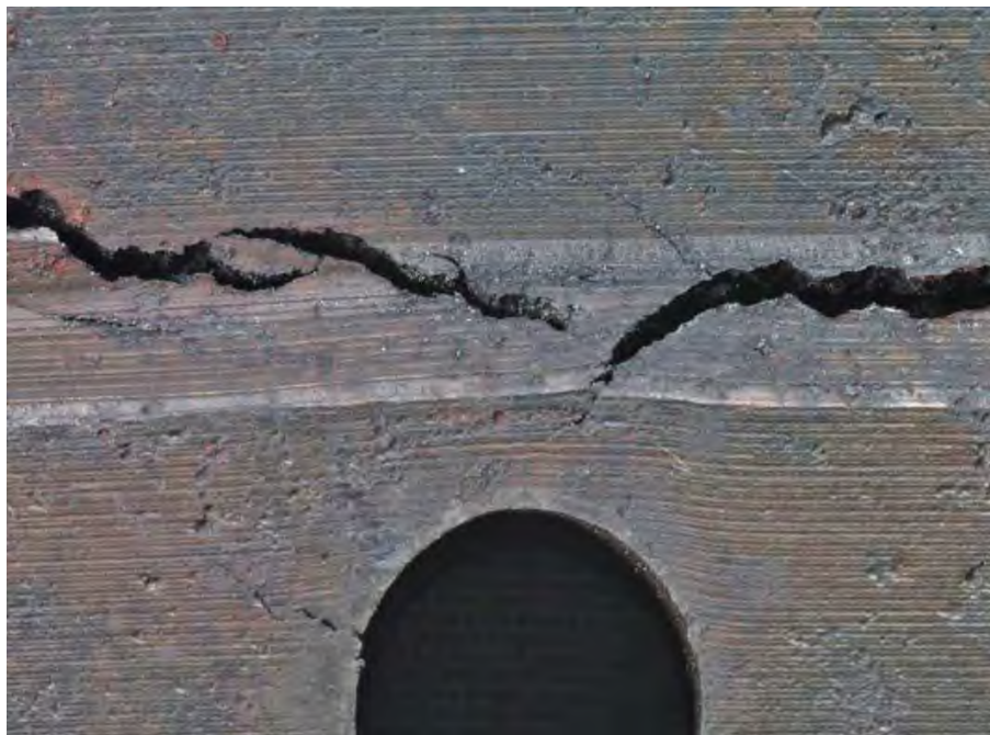
Fig 163. Close-up of SID 14875 subsegment "C4" crack No. 2 shown in Fig. 161, viewed from inlet side.
