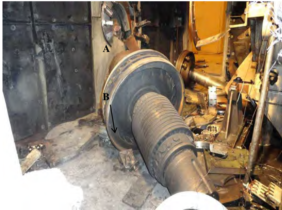
Fig. 105. Photograph of portion of fractured generator shaft shown in Fig. 104.
