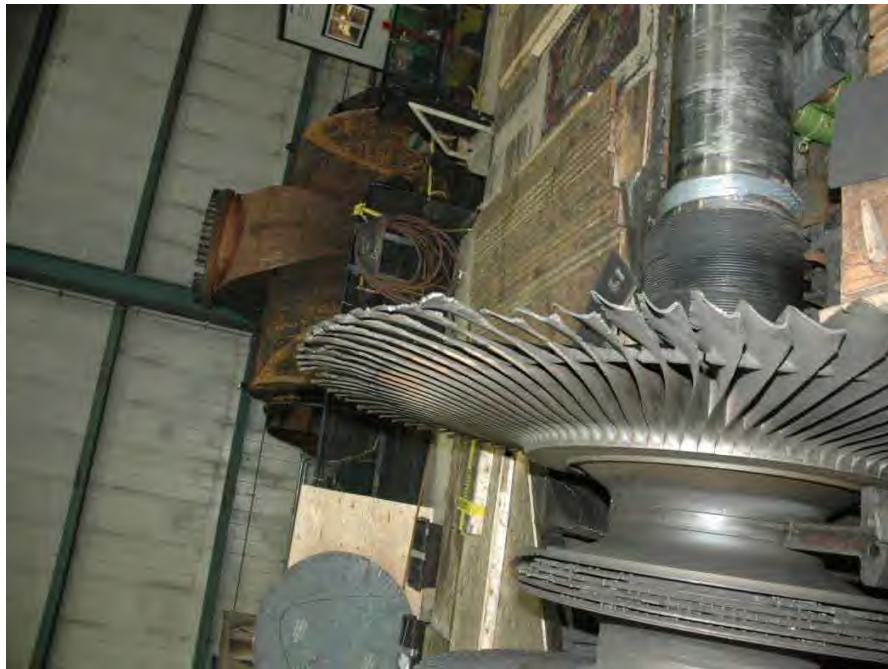
Fig. 63. Close-up photograph of turbine end of low pressure turbine "B" showing extent of damage to last stage blades.
