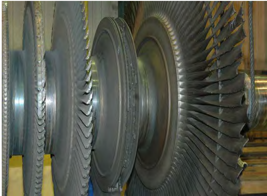
Fig. 67. Photograph of turbine end of low pressure turbine "B" rotor showing missing covers on L-2 and L-3 stage blades.
