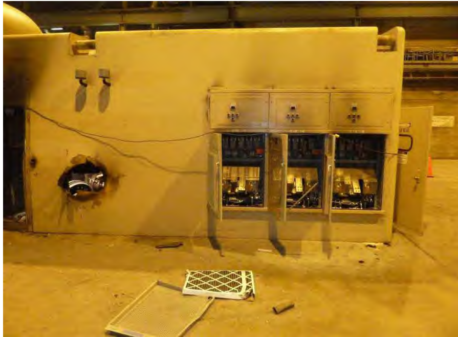
Fig. 8. Photograph of exciter "Doghouse" from Sherco Unit 3 steam turbine generator after event of November 19, 2011.
