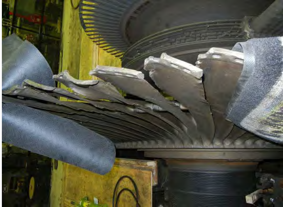
Fig. 64. Photograph of turbine end last stages blades from low pressure turbine "B" showing missing blade spacers.
