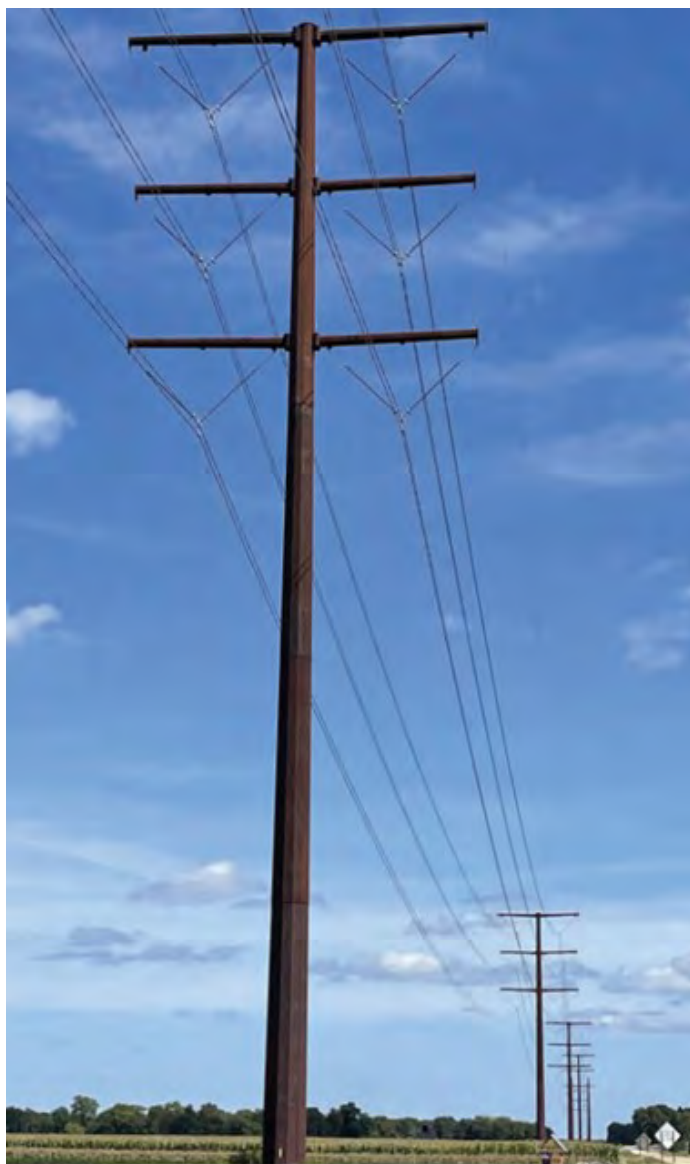
115 kV Steel Double-Circuit Monopole Structure: Brown/Weathering Steel
