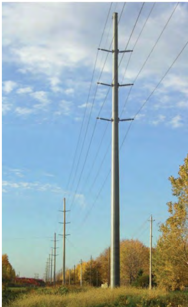
115 kV Steel Double-Circuit Monopole Structure: Silver/Galvanized Steel
