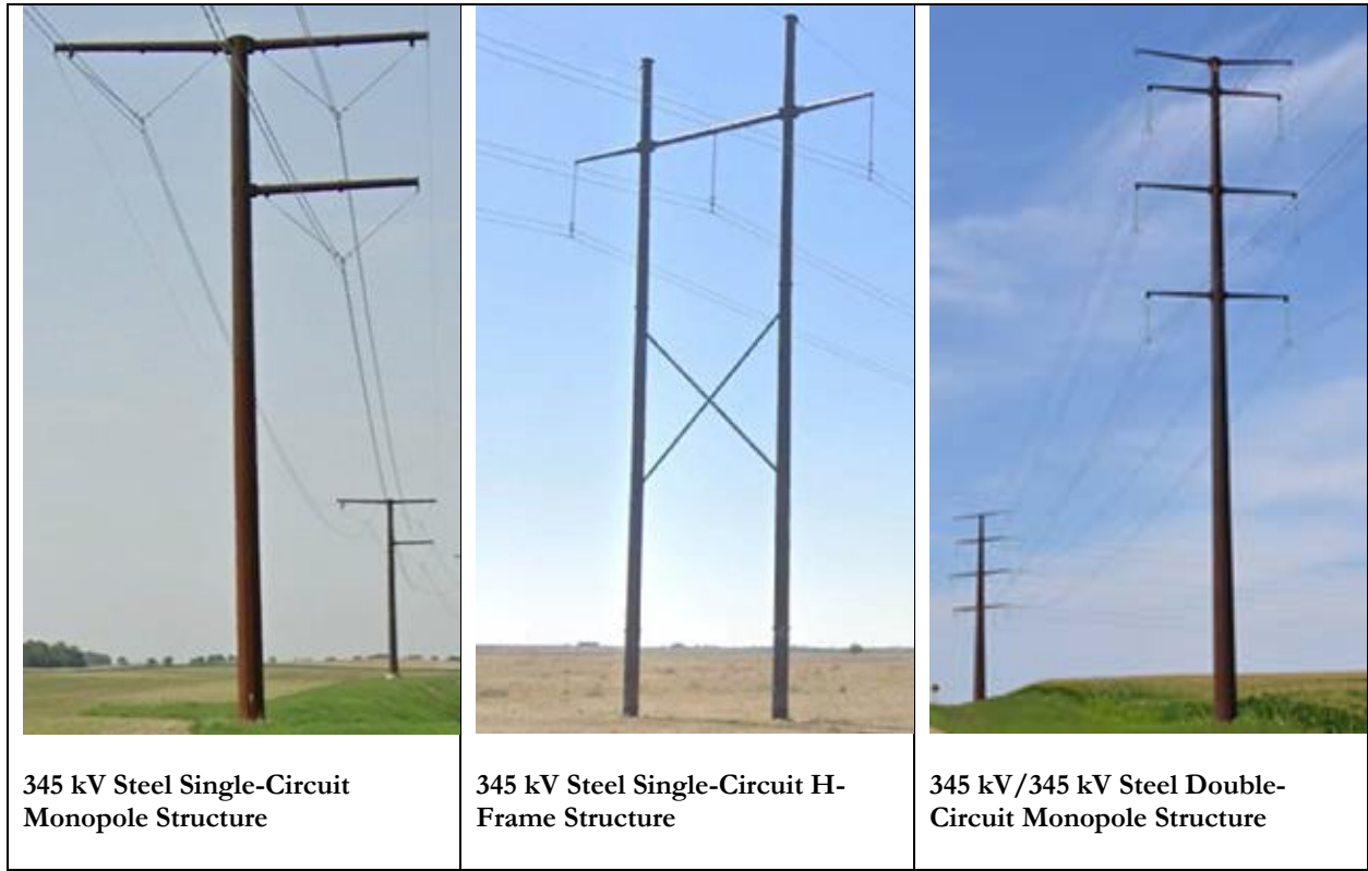
Figure 2.5-2 Typical 345 kV Structures
