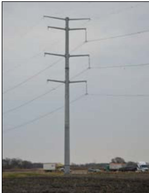
Figure 2.5-3 Existing 345 kV Double-Circuit Capable Monopole Structure with Single Circuit Strung
