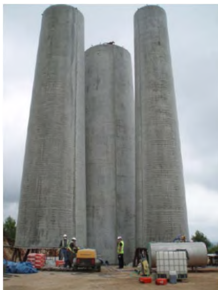
Figure 3-3 AW3000 concrete tower segments
