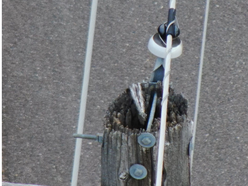
Figure A2 - 2: Example Drone Photo – Wood Pole with Decayed Top
