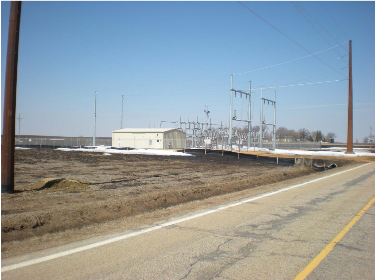
Figure 3: Typical Great River Energy Breaker Station
