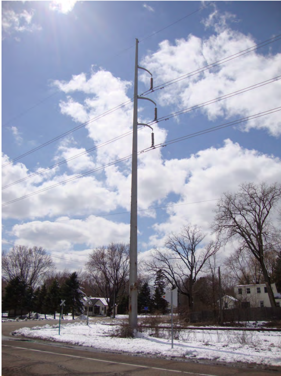
Figure 7. Existing Single Circuit 115 kV Structure 42
