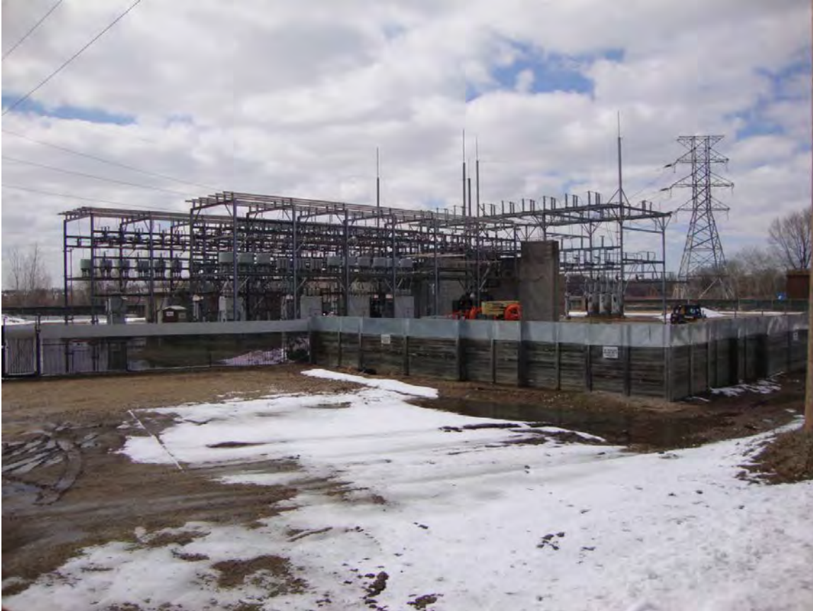
Figure 5. Goose Lake Substation
