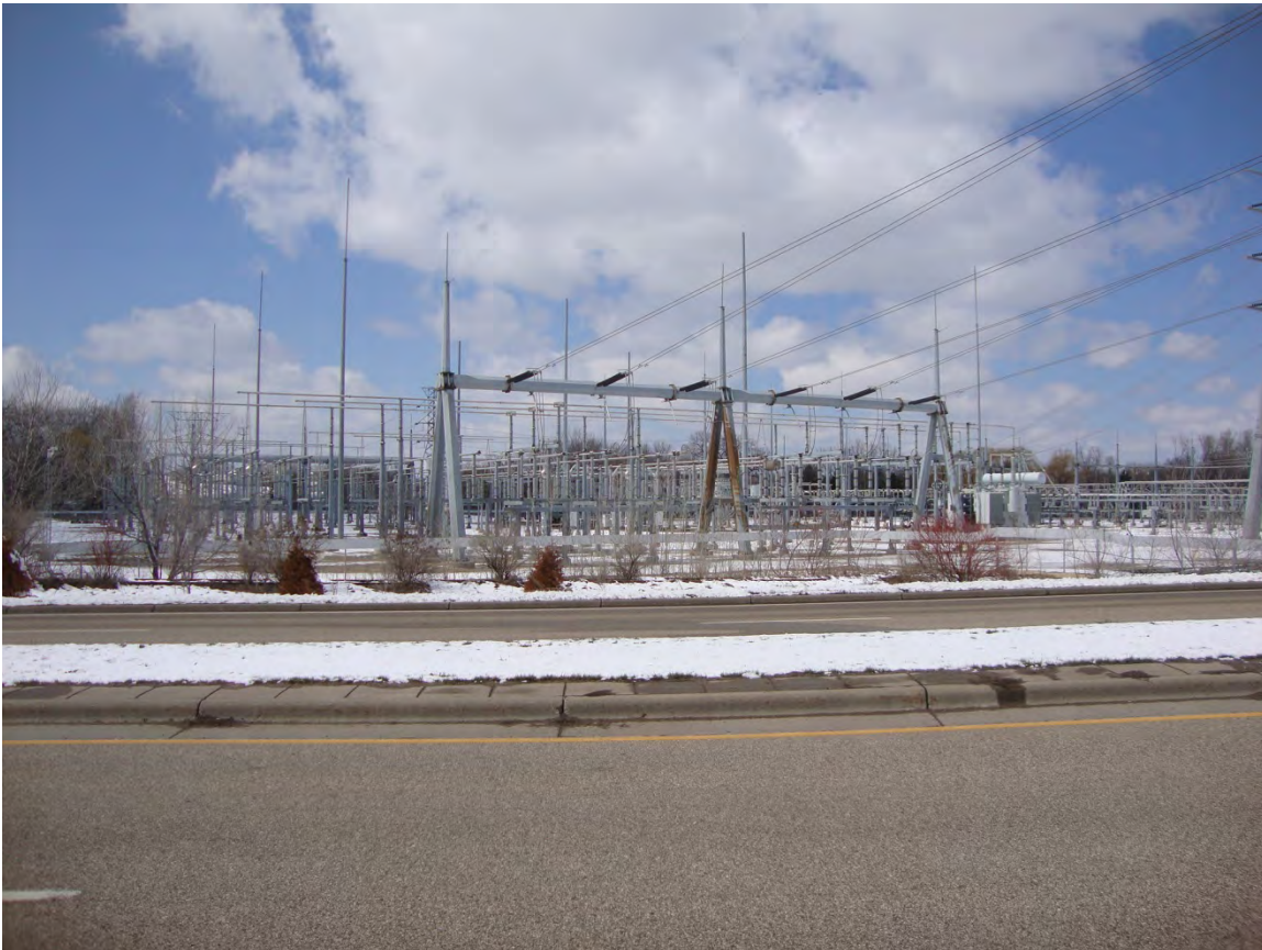
Figure 3. Kohlman Lake Substation
