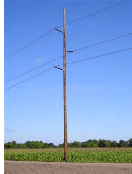
Typical 115-kV wood single circuit structure
