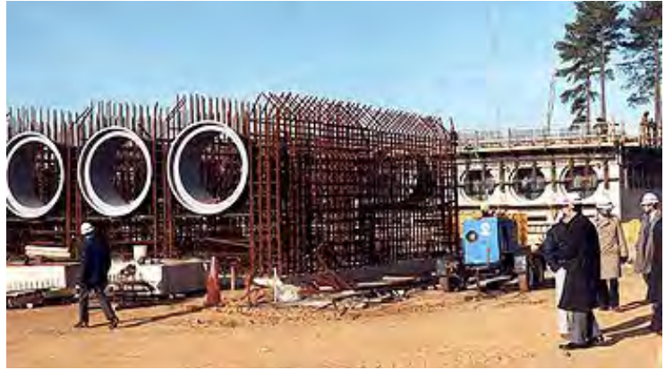
NUHOMS horizontal spent fuel storage system under construction at the Calvert Cliffs Nuclear Power Plant in Lusby, MD.
