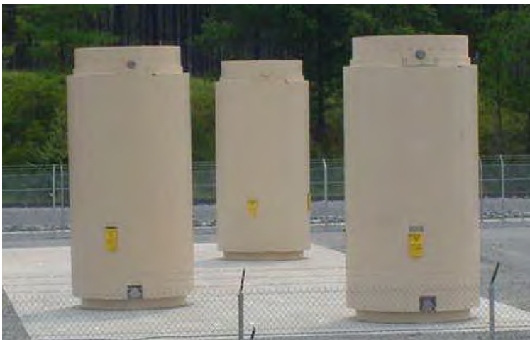
Transportable spent fuel storage casks sit on a storage pad. (Courtesy: Holtec International)
