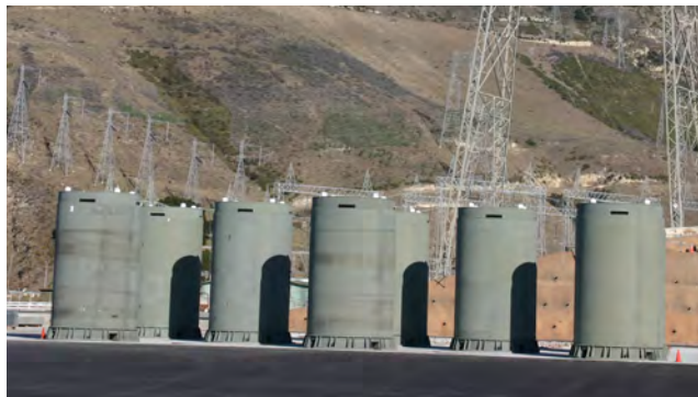
Loaded vertical HI-STORM 100 casks are storing spent fuel at the Diablo Canyon Power Plant in Avila Beach, CA.
