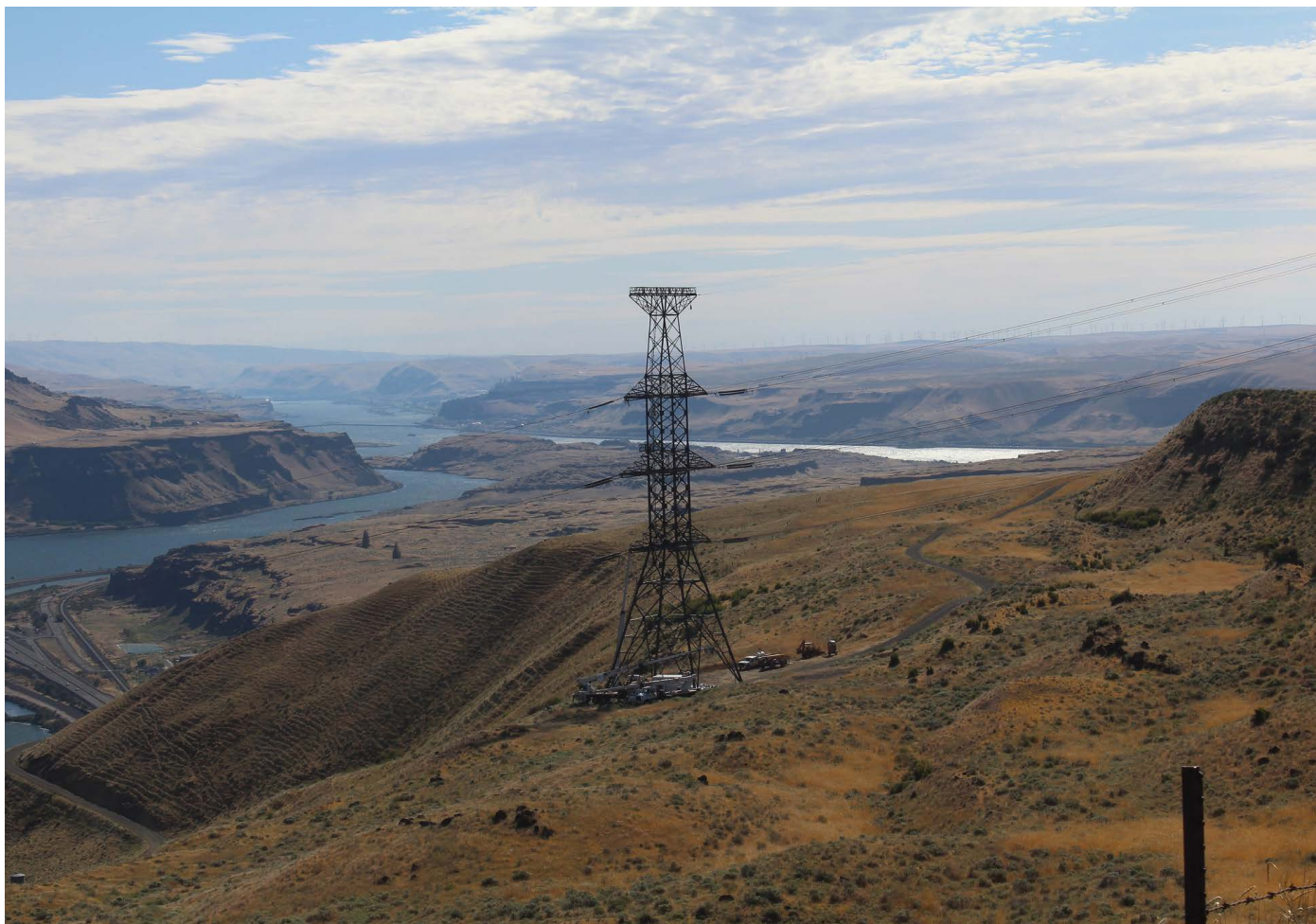
FIGURE 7: Big Eddy-Knight Transmission Line
