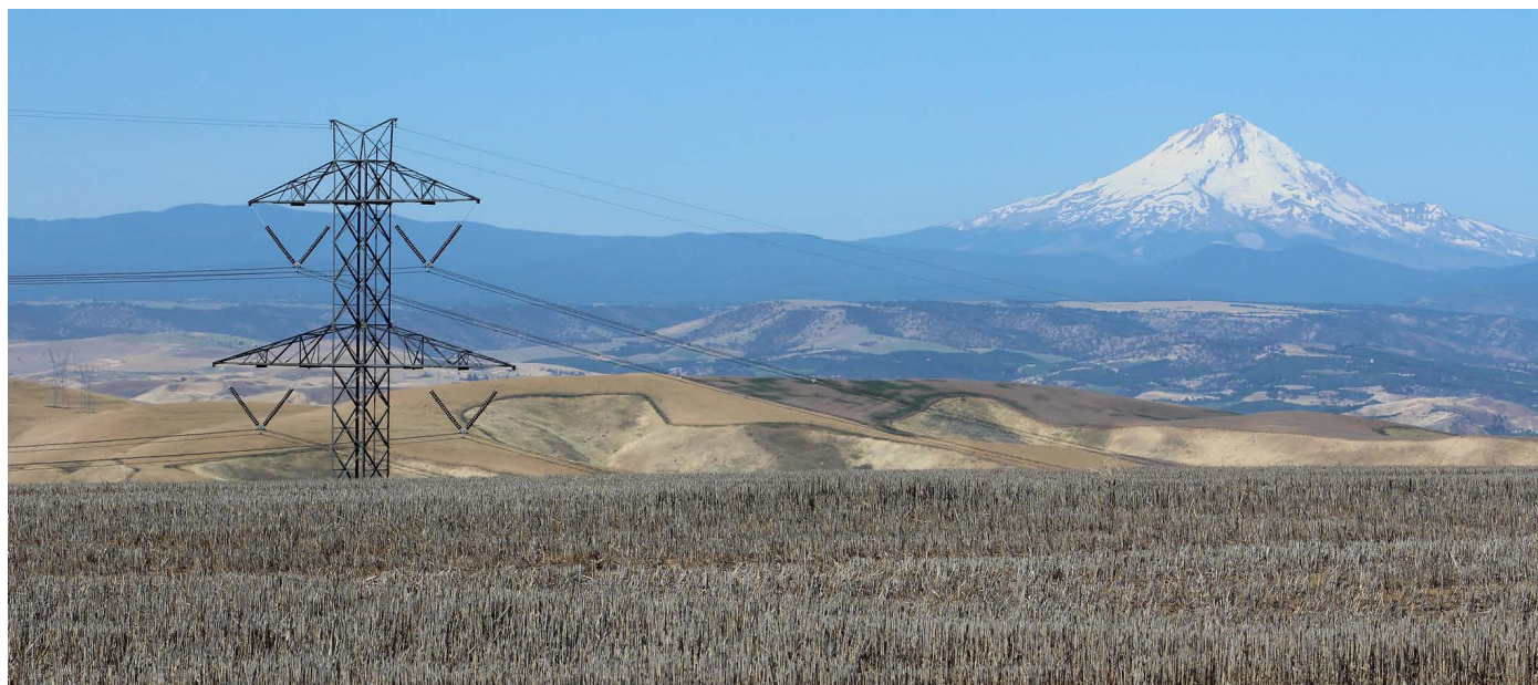
FIGURE 3: Big Eddy-Knight Transmission Line
