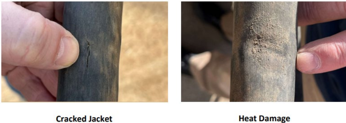
Figure 3 – Control Cable Jacket Defects 86
