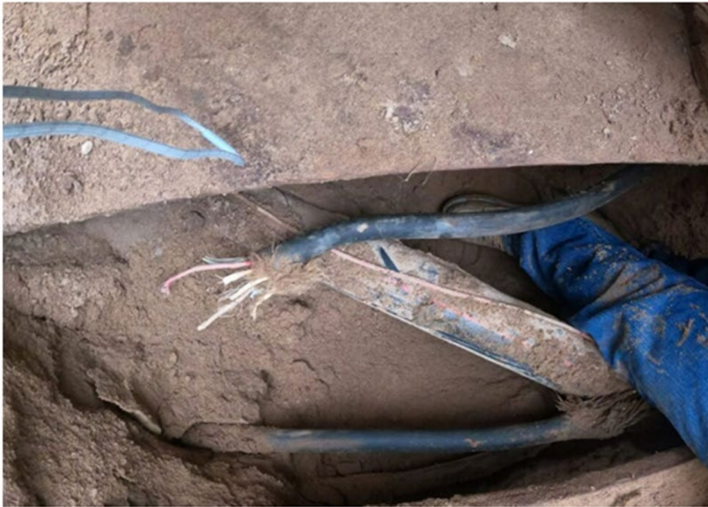
Figure 1: Photograph of Damaged Cables
