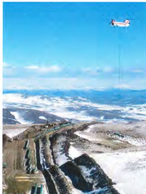
Ruby Pipeline used reduced construction right-of-way and still segregated topsoil in rugged terrain, showing that the Plan requirements can be met safely.
