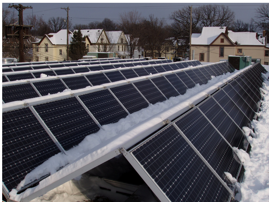
Photo: Minneapolis, MN (40 kW, 2010)
