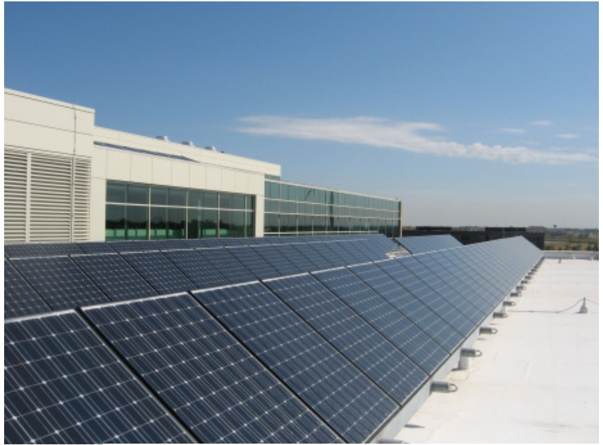
Photo: Maple Grove, MN (72 kW, 2009) Photographer: Ralph Jacobson
