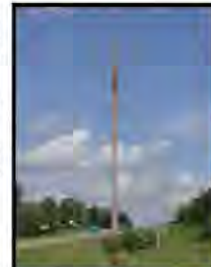
Typical 115 kV Wood Double Circuit Structure
