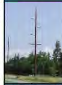
Typical 115 kV Wood Structure with Distribution Underbuild
