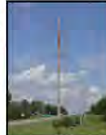
Typical 115 kV Wood Double Circuit Structure
