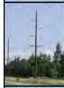
Typical 115 kV Wood Structure with Distribution Underbuild
