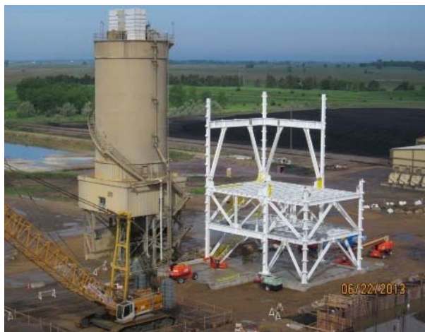
06-22 Waste ash/pebble lime silo
