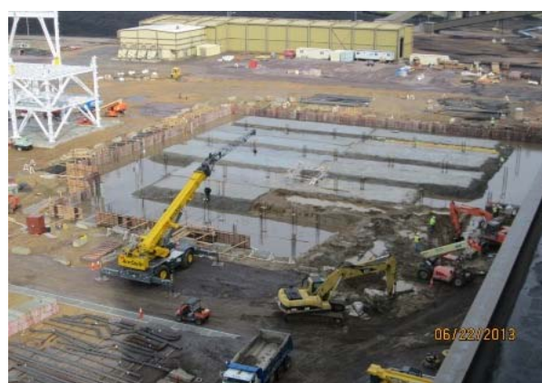
06-22 Baghouse SW view
