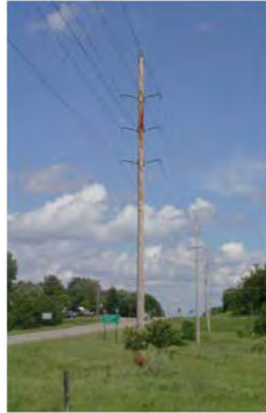
Typical Double Circuit 115 kV Structure
