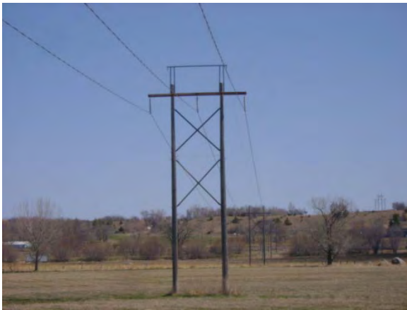
Typical H-Frame 115 kV Structure
