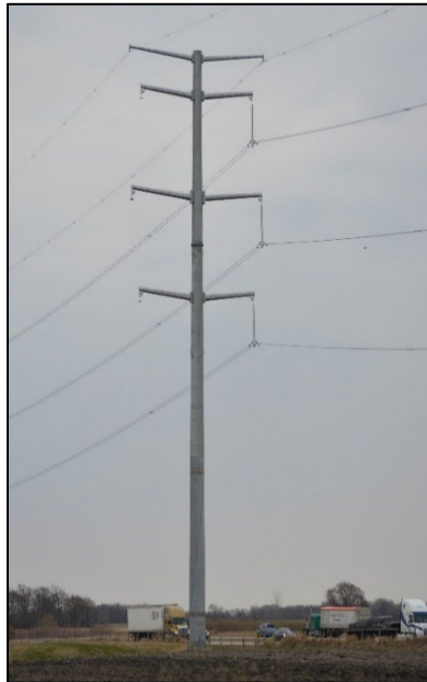
Figure 2-1 Existing 345 kV Structures on Eastern Segment
