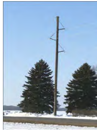
Typical Braced Post 115 kV Structure
