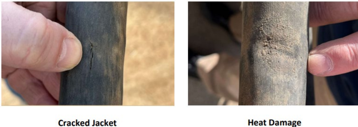
Figure 3 – Control Cable Jacket Defects 68
