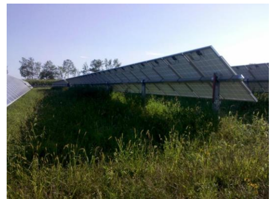
Figure 3. Typical Solar Array
