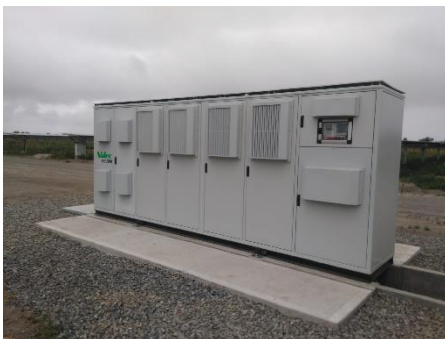
Figure 5: Typical Inverter Skid
