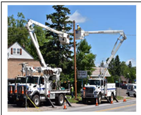
Minnesota Power Crews in Action. The restoration efforts were recognized by EEI. The Company received the Emergency Recovery Award for performance following the July 2016 wind storm event.
