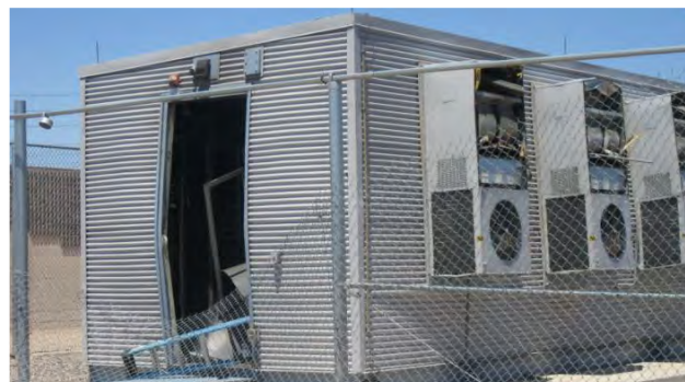
Figure 3: BESS Exterior after event (image credit: APS)
