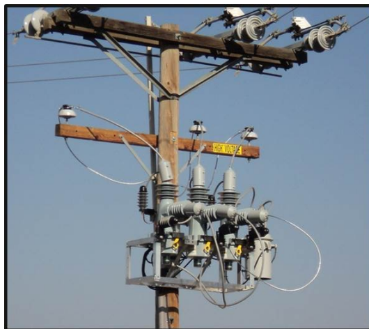
Figure 4: Recloser on a Distribution Pole
