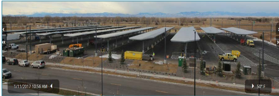
Figure 10: 1.3 MW Carport Solar Installation
