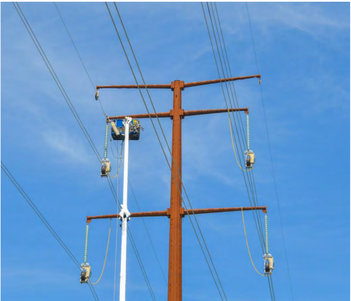
Figure 4. Double-Circuit 345 kV Image
