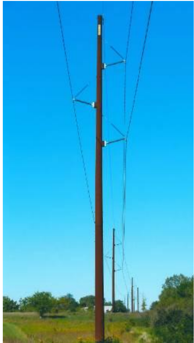
161 kV Single Circuit
