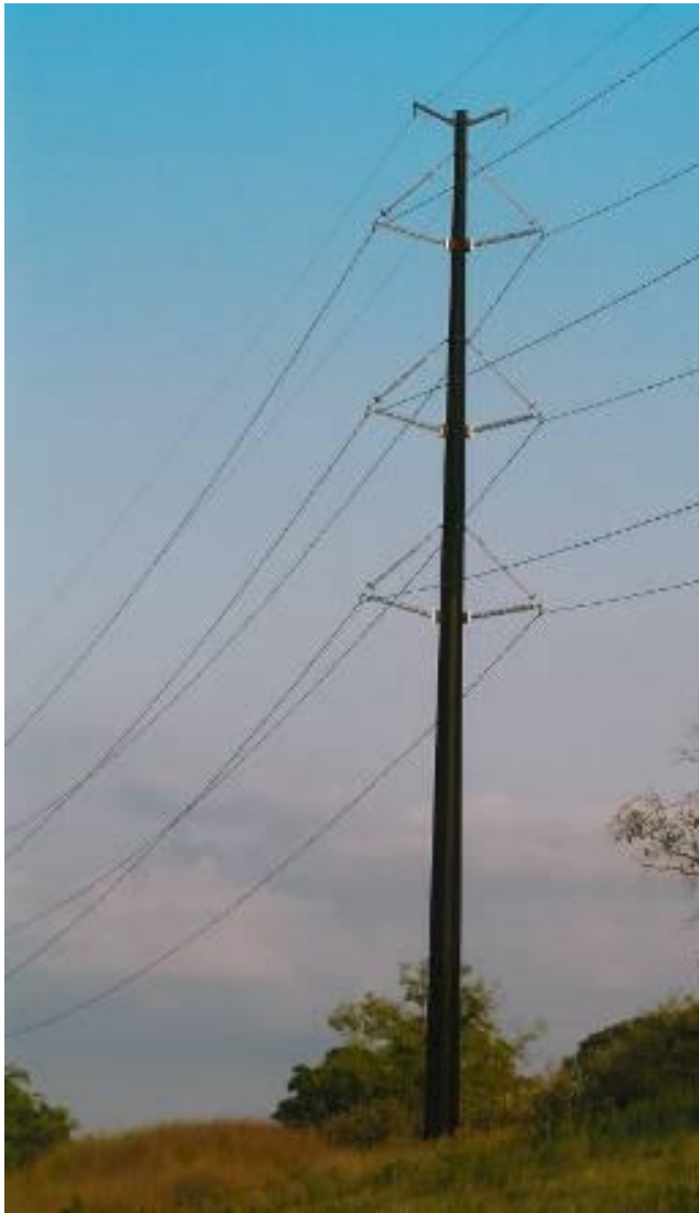
161/161 kV Double Circuit
