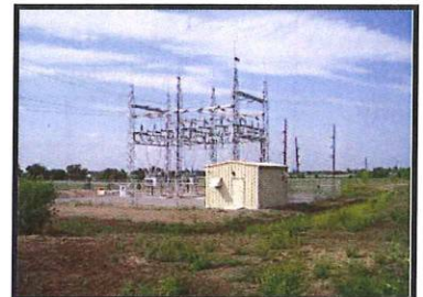
Typical Transmission Breaker Station
