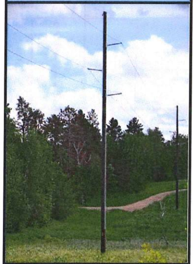
Typical 115 kV Wood Transmission Structure
