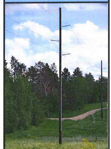
Typical 115 kV Wood Transmission Structure
