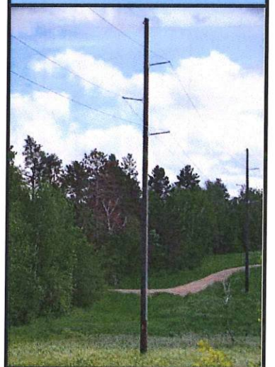
Typical 115 kV Wood Transmission Structure
