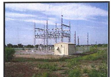
Typical Transmission Breaker Station
