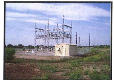
Typical Transmission Breaker Station
