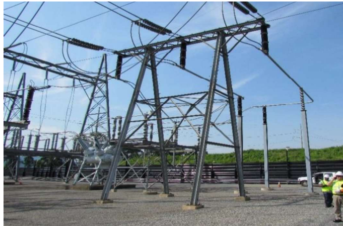
Image 3: Typical A-Frame Deadend Structure
