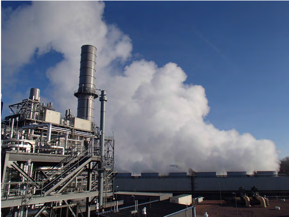
Figure 9. Water Vapor Plumes at Mankato Energy Center 104
