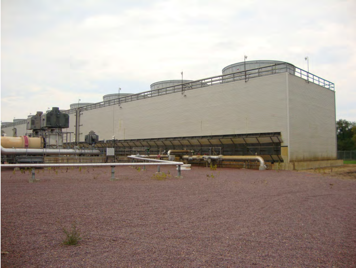
Figure 6. Existing Cooling Tower at Mankato Energy Center 69
