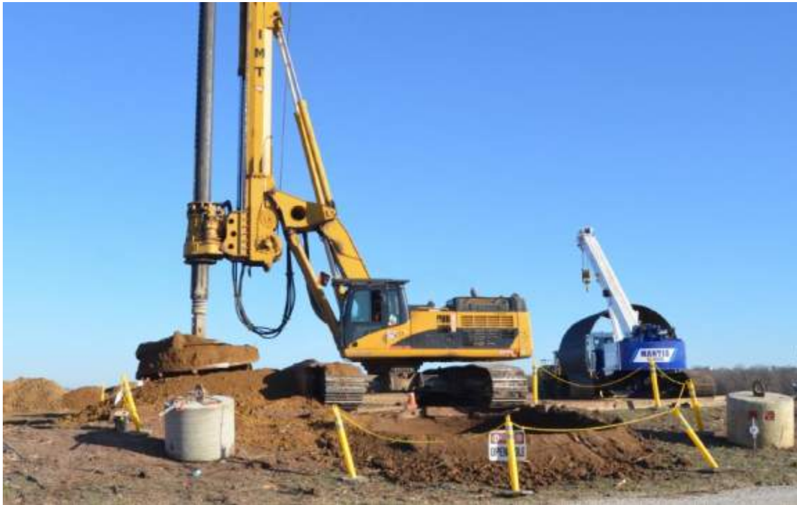
The diameter and depth of the hole depend on structure design and soil conditions Source: reference (7)
