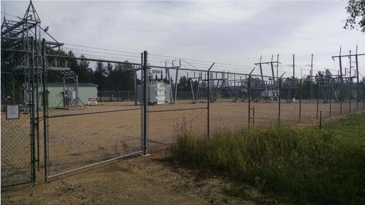
Figure 6. Dog Lake Substation 63
