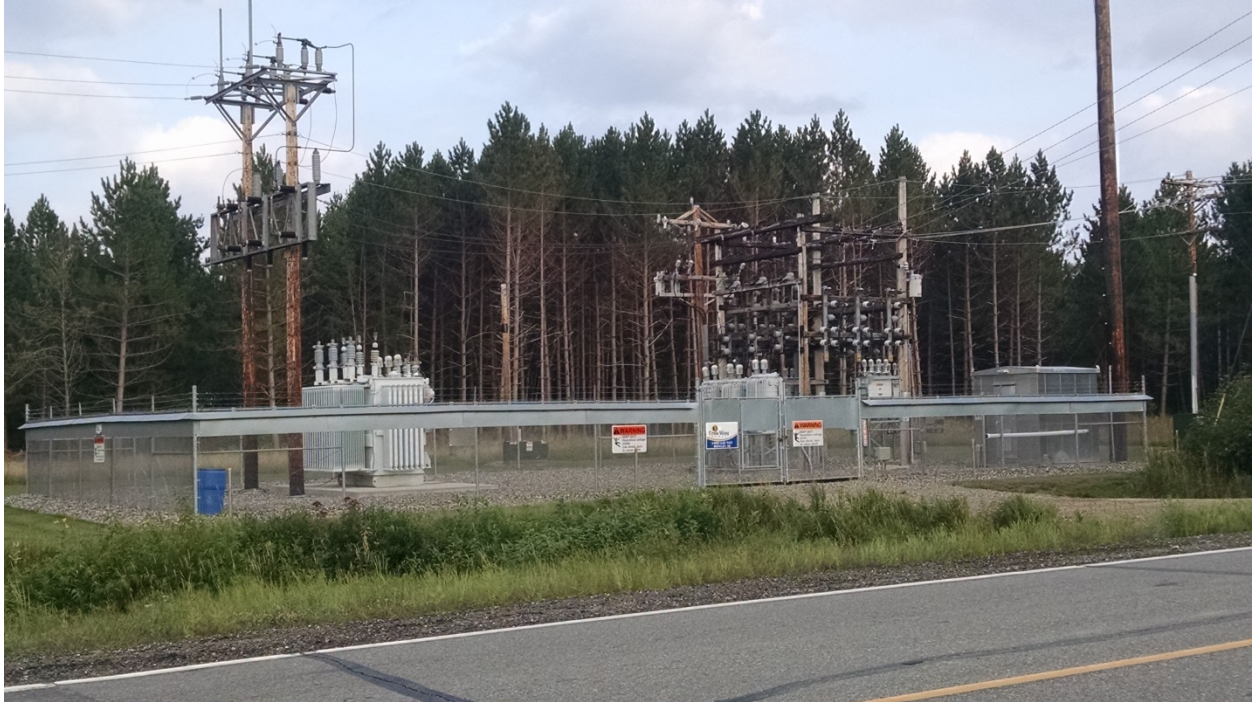
Figure 5. Existing Motley Substation 60
