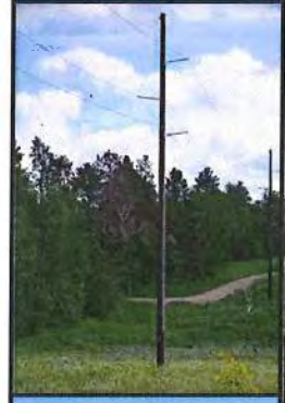
Typical 115 kV Wood Single Circuit Structure
