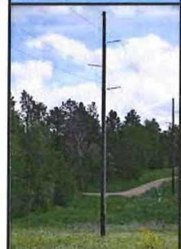
Typical 115 kV Wood Single Circuit Structure
