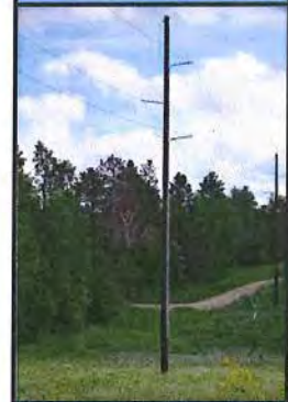
Typical 115 kV Wood Single Circuit Structure
