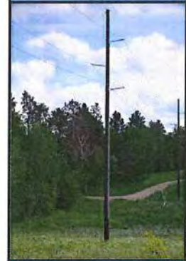
Typical 115 kV Wood Single Circuit Structure
