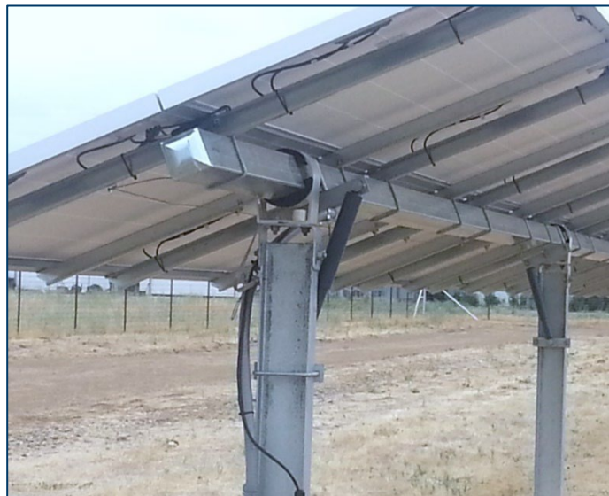
Figure 3 Tracking System and Foundation Posts
