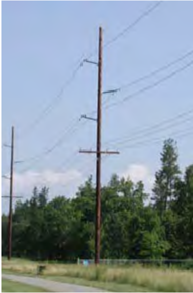
Typical Single Circuit Structure with Distribution Underbuild
