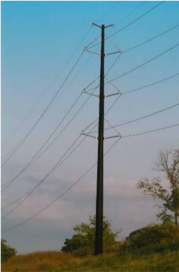
161 kV/161 kV Double-Circuit
