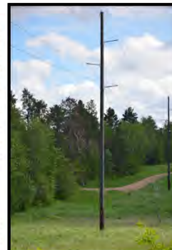
Typical 115 kV Wood Transmission Line Structure
