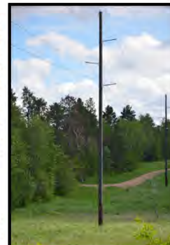
Typical 115 kV Wood Transmission Line Structure
