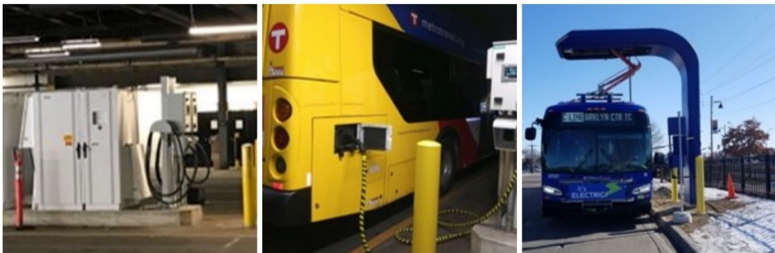
Figure 2. Example of Metro Transit Charging Equipment
